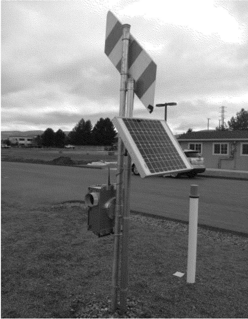
Installed Remote Methane Leak Detector at PG&E [Redacted] (February 2013)
