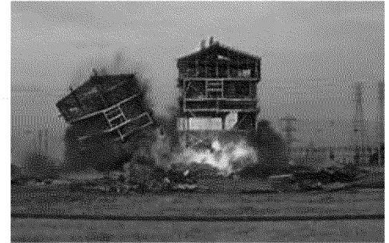
2012 & 2013 Kern Power Plant Incidents
