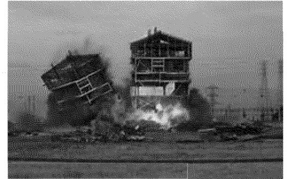
2012 & 2013 Kern Power Plant Incidents
