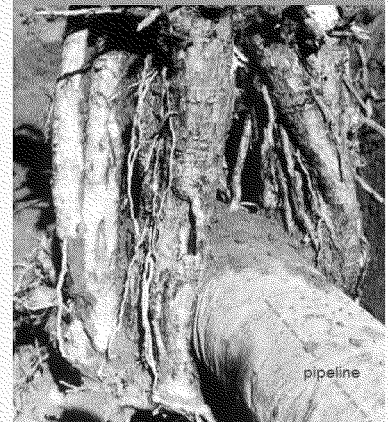
Example of the impact tree roots can have on a pipeline.
