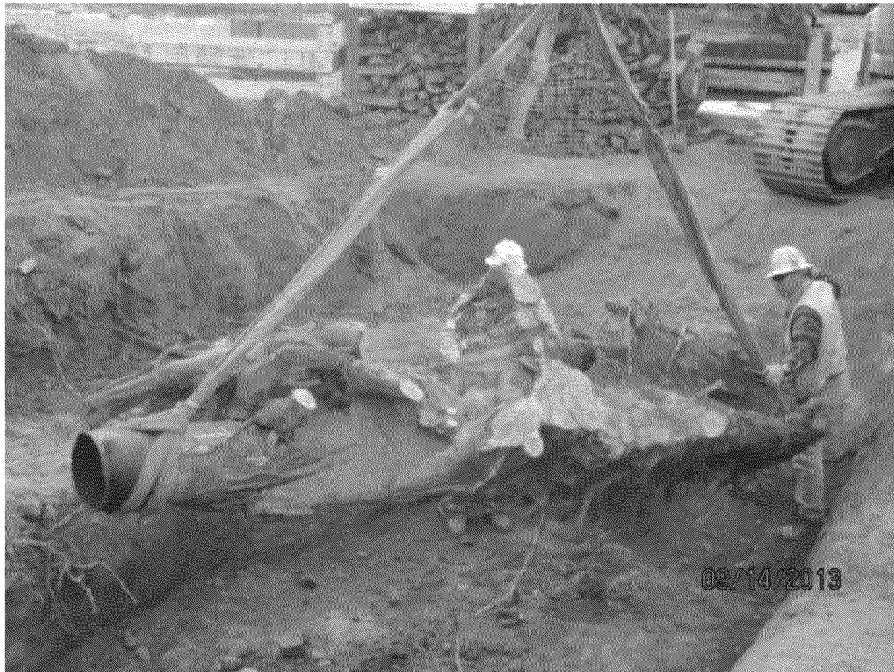
Figure 6. RWVIM-90-13 (Hall Road)
