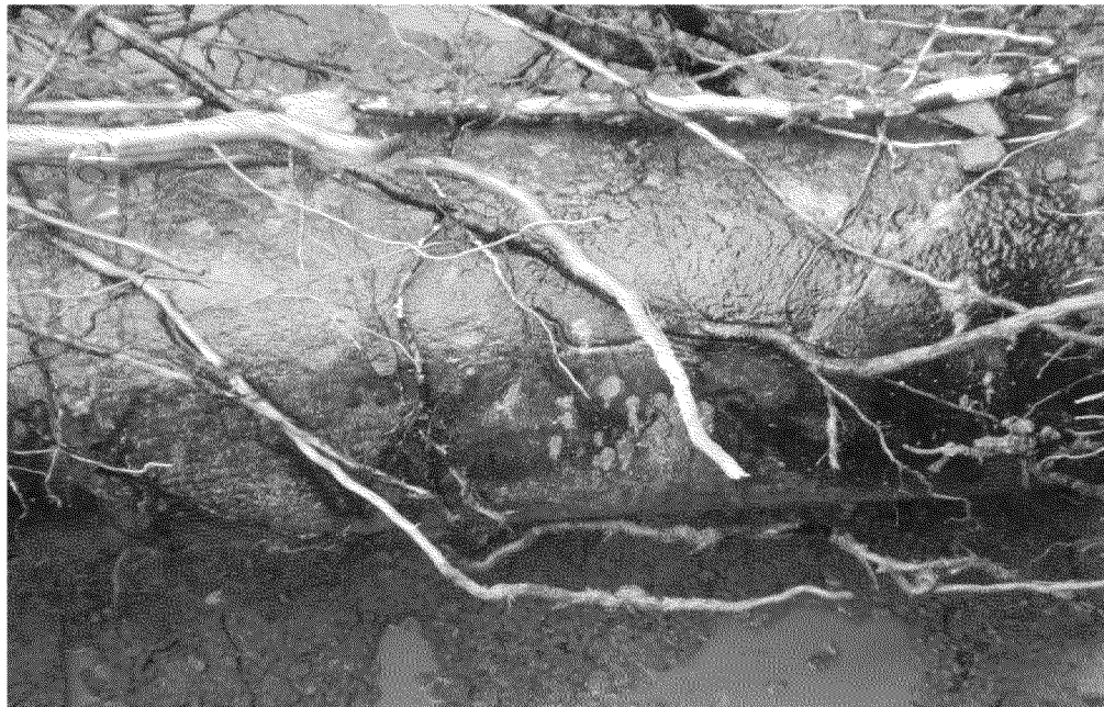
Figure 4. RWVIM-74-13 (Atascadero) (Tape coating damage)
