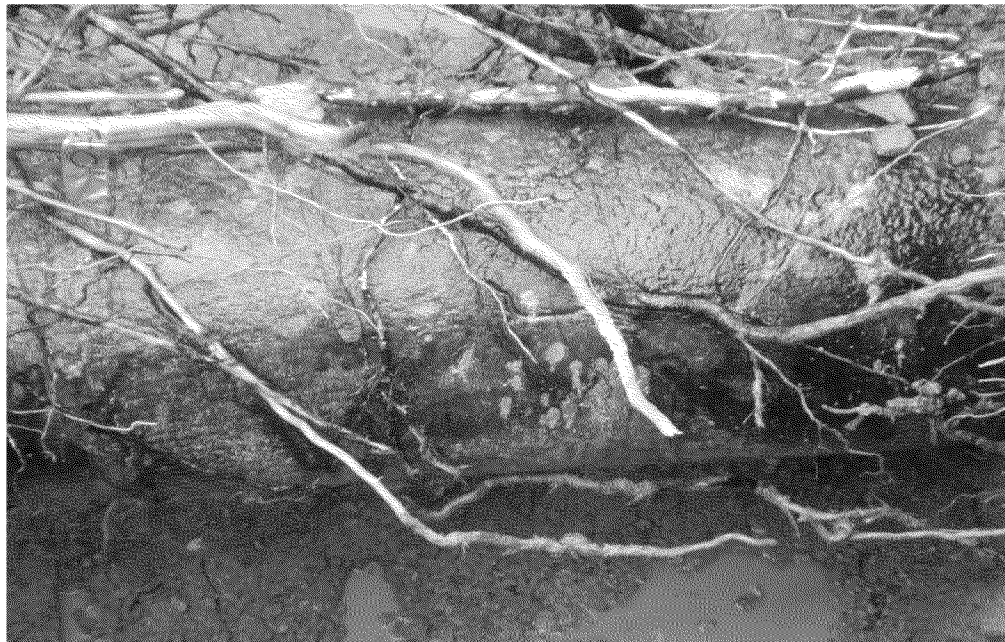
Figure 4. RWVIM-74-13 (Atascadero) (Tape coating damage)
