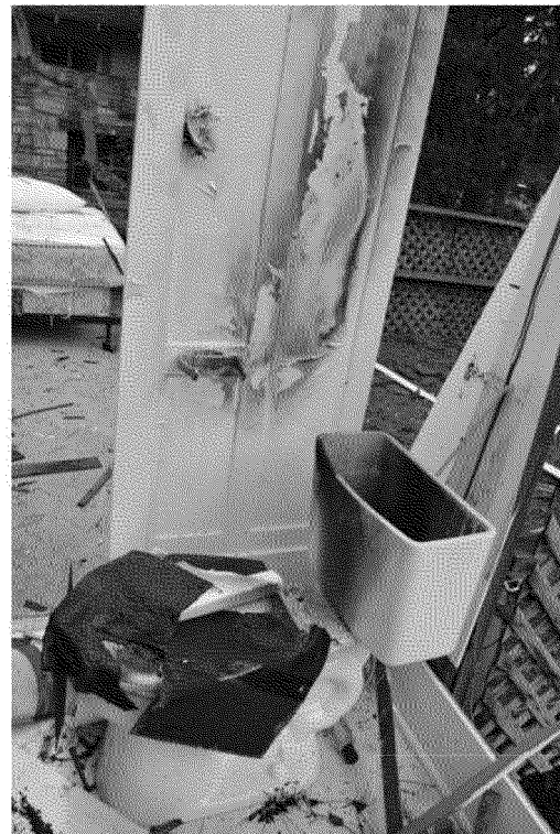
Figure 14. Bathroom toilet. Photograph by Exponent on March 6, 2014.
