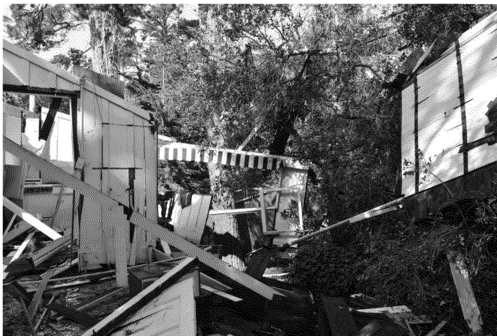
Figure 10. Incident house looking West into the laundry room. Roof section on right side of picture. Photograph by Exponent on March 4, 2014.
