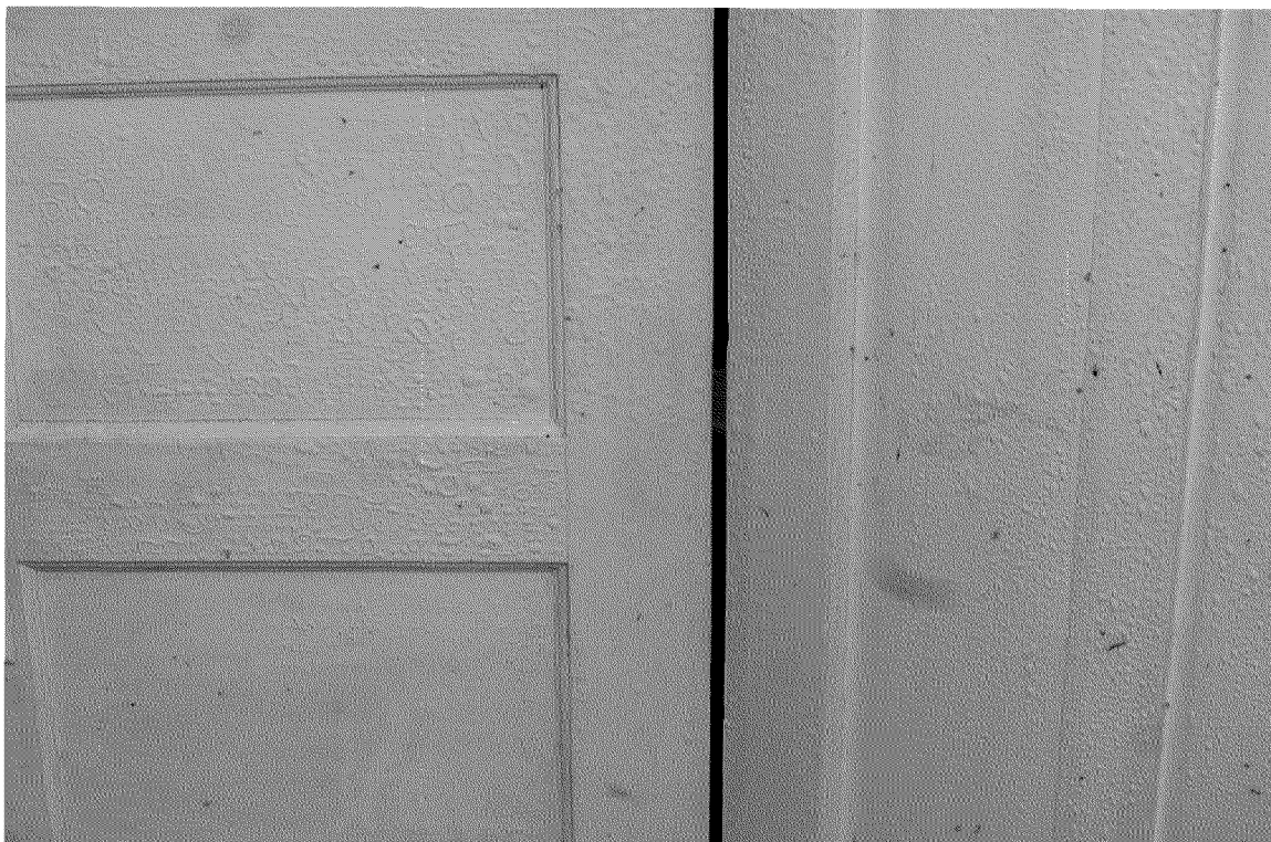
Figure 12. Close-up of the paint blistering on bedroom wall and door. Photograph by Exponent on March 7, 2014.
