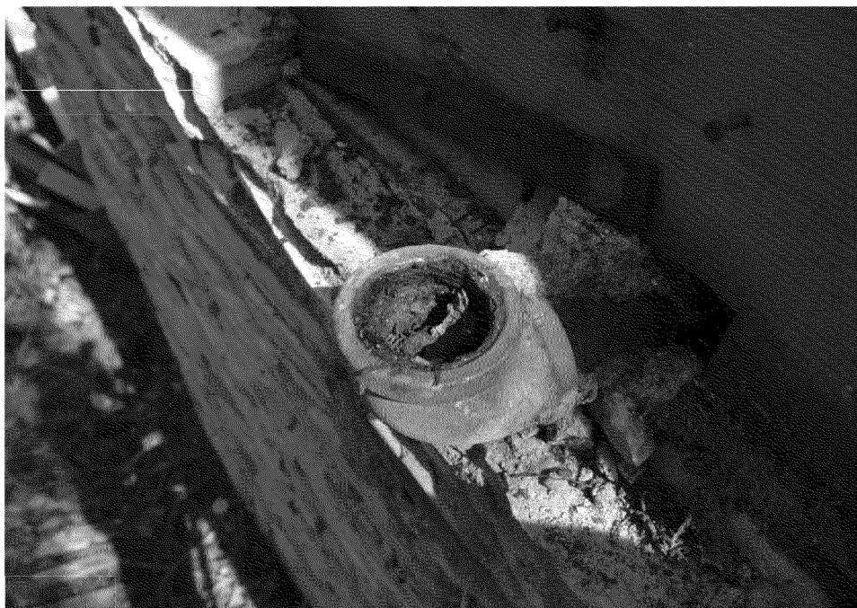
Figure 19. Vent pipe (broken off) in the bathroom. Vent pipe likely broken off during the explosion. Photograph by Exponent on March 7, 2014.
