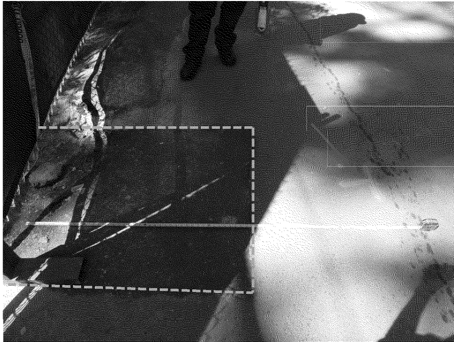
Figure 35. Relative location of cold asphalt patch for gas service tee (dashed yellow lines) and sewer lateral tap connection to sewer main (green arrow) for subject residence. Residence is to the left in photograph. Photograph by Exponent on March 11, 2014.
