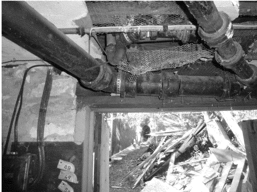
Figure 41. Multiple connections to building sewer system inside residence. Arrow indicates tub plumbing trap. Photograph from inside residence's basement. Photograph by Exponent on March 11, 2014.
