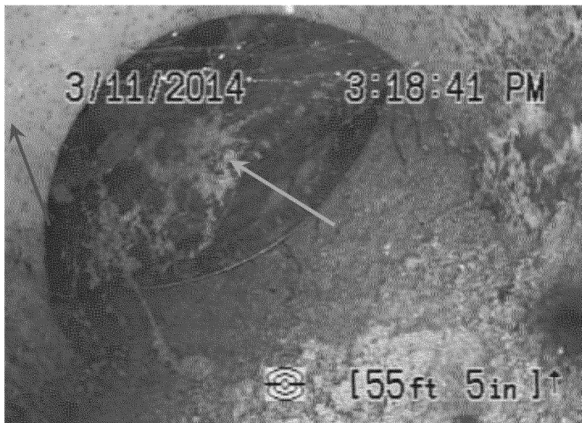
Figure 43. Sewer lateral joint offset at connection between white plastic pipe segment (green arrow) and apparent cast iron pipe (yellow arrow). Source: FES.
