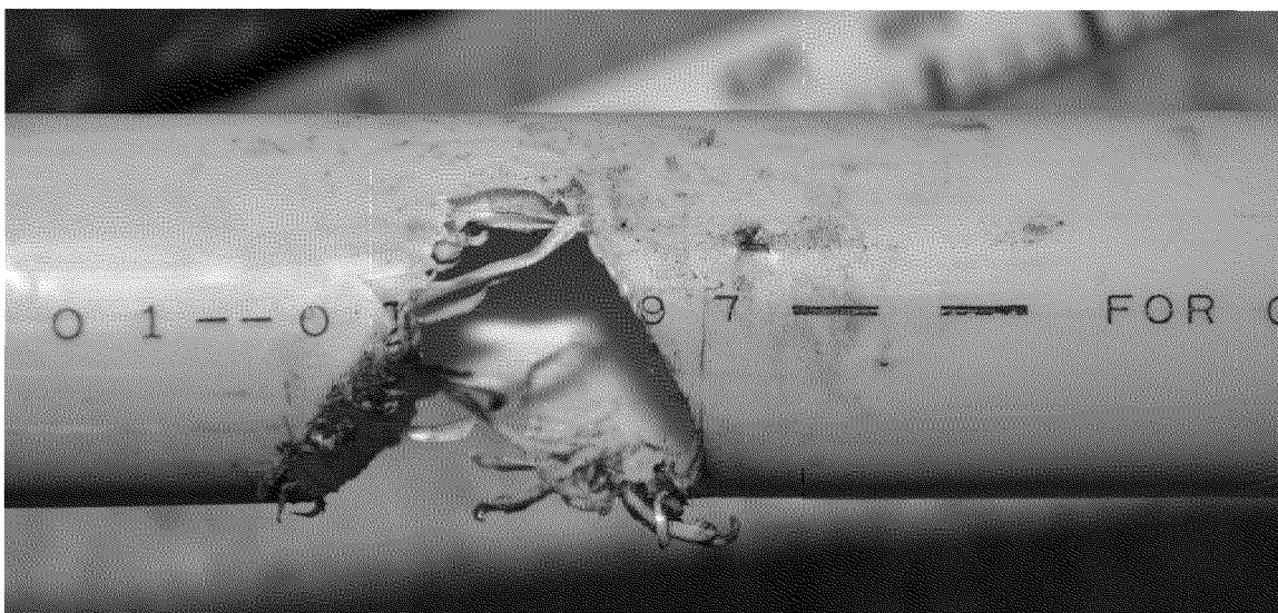
Figure 30. Close-up of the visible portion of the date code on the plastic pipe. Photograph by Exponent on March 10, 2014.
