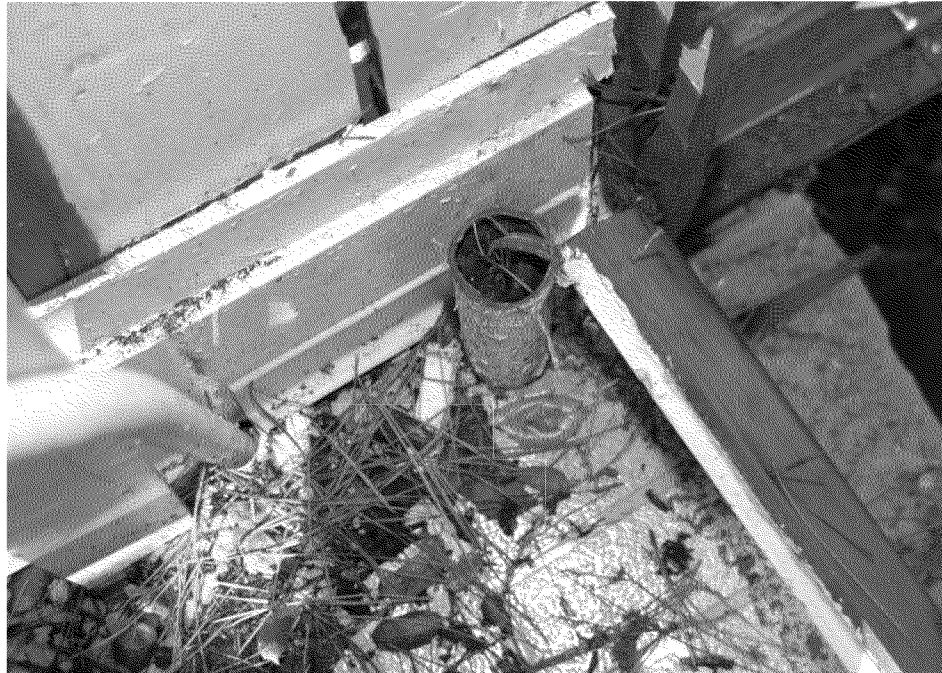
Figure 18. Sewer vent pipe (broken off) in the laundry room. Vent pipe likely broken off during the explosion. Photograph by Exponent on March 7, 2014.
