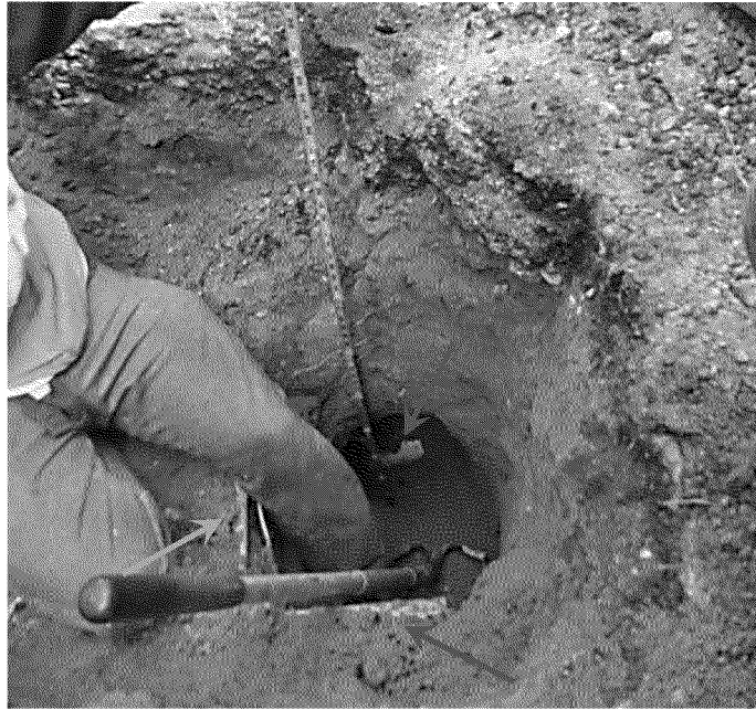
Figure 45. Excavation to expose sewer lateral at subject residence in the vicinity of gas service tee. Yellow arrow indicates gas main along 3 rd Avenue. Red arrow indicates gas service line. Green arrow indicates sewer lateral. Photograph by Exponent on March 21, 2014.
