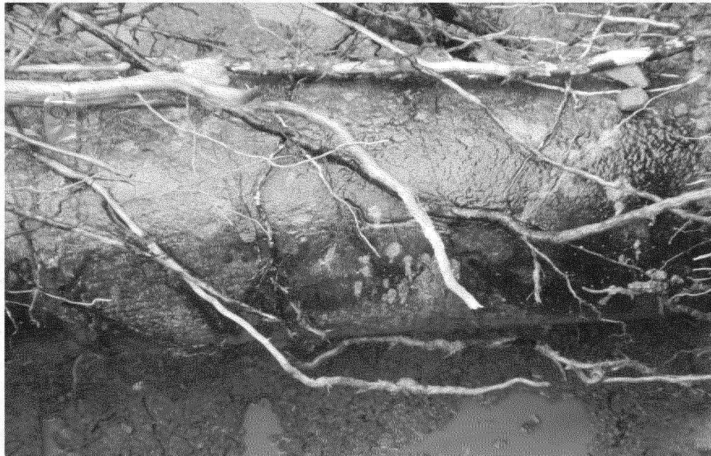
Figure 4. RWVIM-74-13 (Atascadero) (Tape coating damage)
