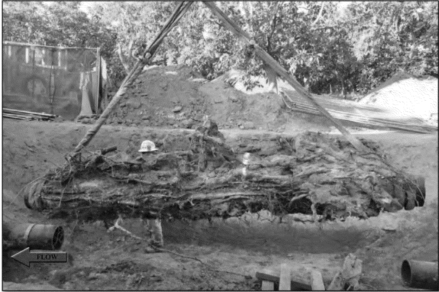
A 15-foot section of pipe with roots intact was extracted from the construction site.
