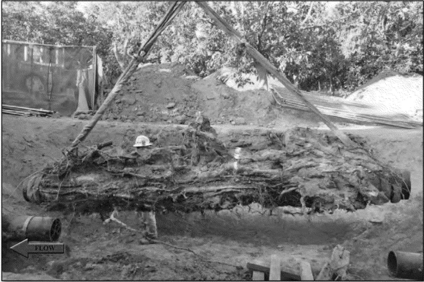
A 15-foot section of pipe with roots intact was extracted from the construction site.
