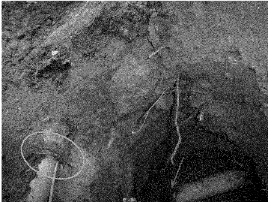
Figure 47. End of annular space in gas main along Redacted (yellow oval) in vicinity of sewer lateral offset joint (green arrow). Photograph by Exponent on March 21, 2014.
