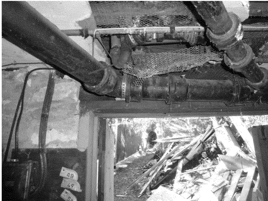
Figure 41. Multiple connections to building sewer system inside residence. Arrow indicates tub plumbing trap. Photograph from inside residence's basement. Photograph by Exponent on March 11, 2014.
