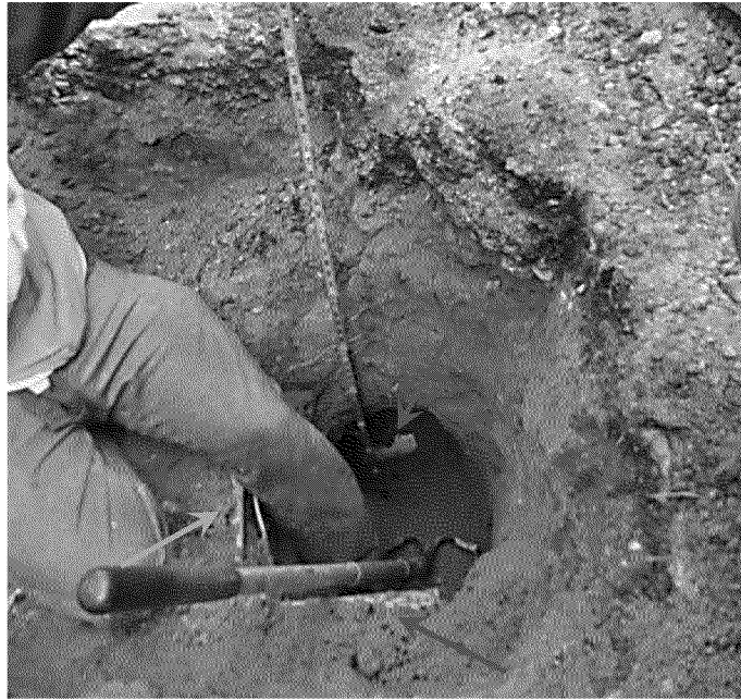
Figure 45. Excavation to expose sewer lateral at subject residence in the vicinity of gas service tee. Yellow arrow indicates gas main along [Redacted] [Redacted] Red arrow indicates gas service line. Green arrow indicates sewer lateral. Photograph by Exponent on March 21, 2014.
