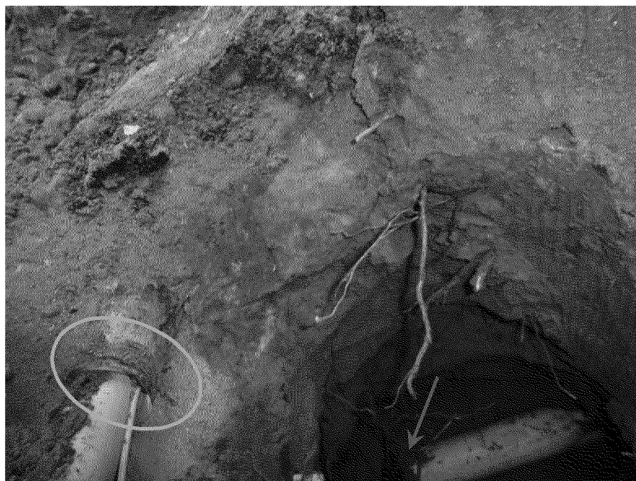
Figure 47. End of annular space in gas main along Redacted (yellow oval) in vicinity of sewer lateral offset joint (green arrow). Photograph by Exponent on March 21, 2014.
