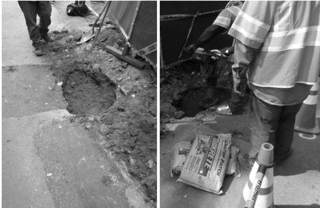
Figure 58. Excavation (left) and re-compaction (right) near gas service tee. Photographs by Exponent on March 21, 2014.
