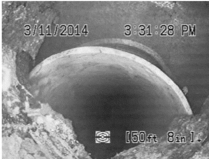
Figure 42. Dislocated joint between an apparently white plastic pipe and cast iron sewer lateral. Source: FES.
