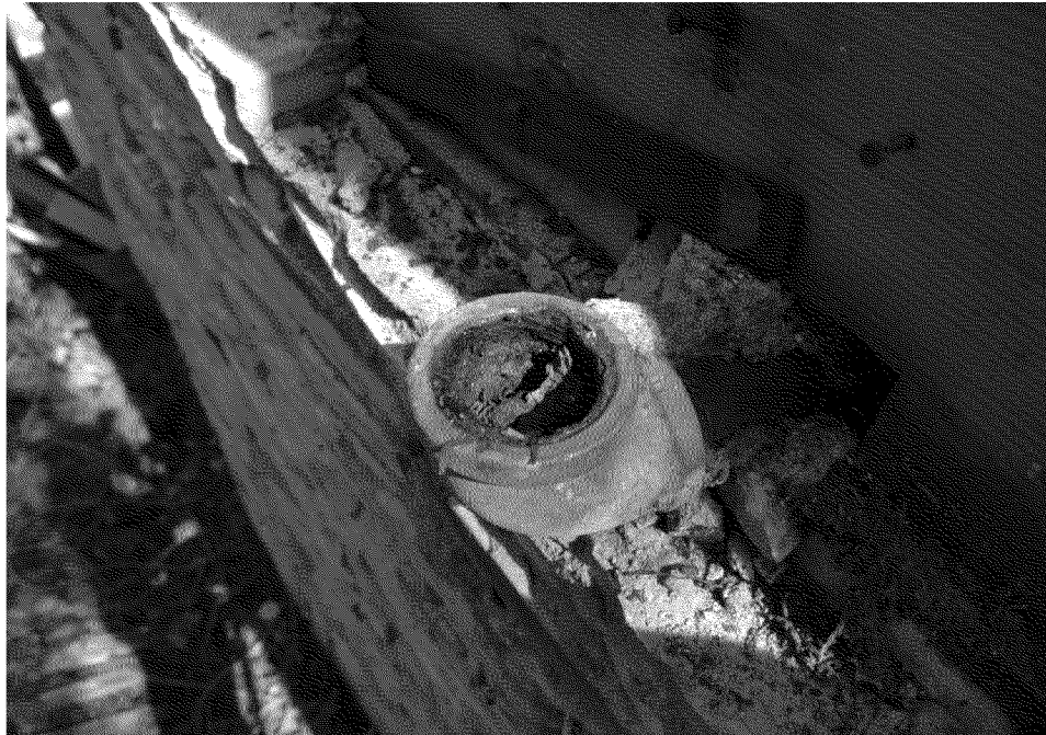
Figure 19. Vent pipe (broken off) in the bathroom. Vent pipe likely broken off during the explosion. Photograph by Exponent on March 7, 2014.
