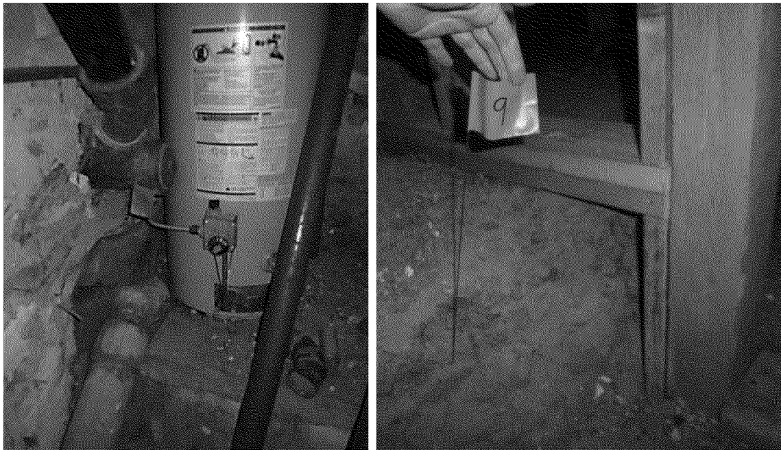
Figure 56. Example monitoring points at the residence's basement. Monitoring point #8 (left) by the cleanout next to water heater. Monitoring point #9 (right) near center of basement, over soil. Photographs by Exponent on March 21, 2014.
