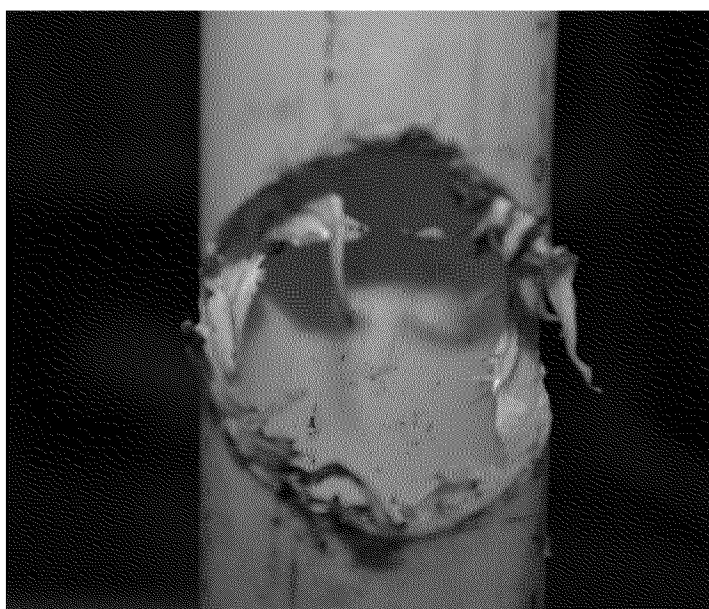
Figure 29. Perforations in plastic gas line: Save-a-Valve fitting (top) and M/2 fitting (bottom). Photographs by Exponent on March 10, 2014.
