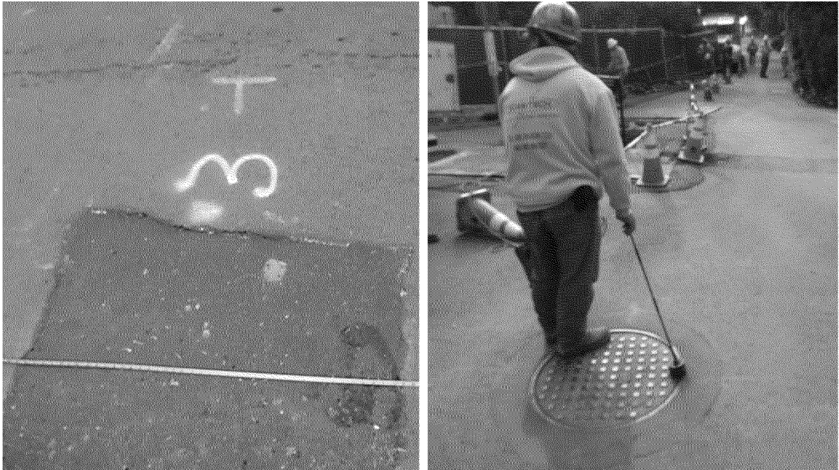
Figure 55. Example monitoring points outside of residence. Monitoring point #3 (left) near excavation performed by PG&E at gas service tee for residence. Monitoring point #19 (right) at sewer manhole [Redacted] [Redacted] Photographs by Exponent on March 21, 2014.
