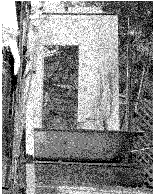
Figure 13. Fire pattern on bathroom wall, looking South from Redacted Photograph by Exponent on March 7, 2014.
