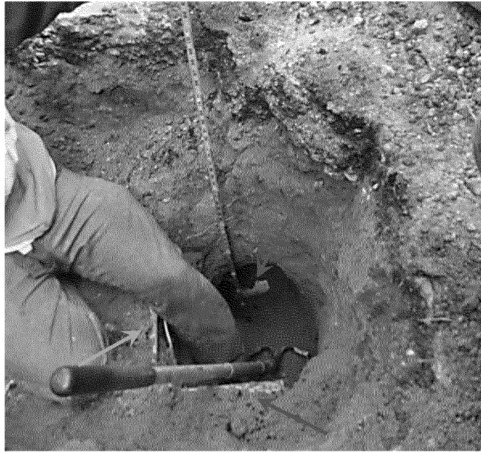
Figure 45. Excavation to expose sewer lateral at subject residence in the vicinity of gas service tee. Yellow arrow indicates [Redacted] [Redacted] Red arrow indicates gas service line. Green arrow indicates sewer lateral. Photograph by Exponent on March 21, 2014.
