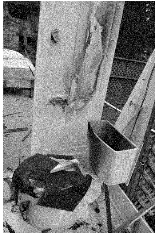
Figure 14. Bathroom toilet. Photograph by Exponent on March 6, 2014.
