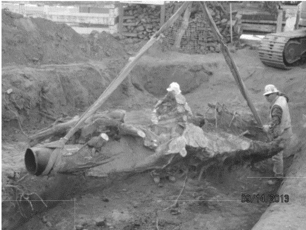
Figure 6. RWVIM-90-13 (Hall Road)
