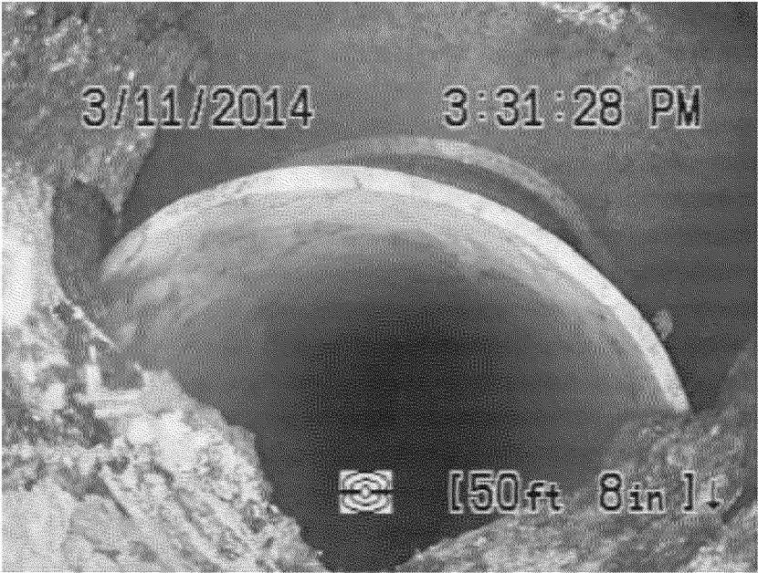
Figure 42. Dislocated joint between an apparently white plastic pipe and cast iron sewer lateral. Source: FES.
