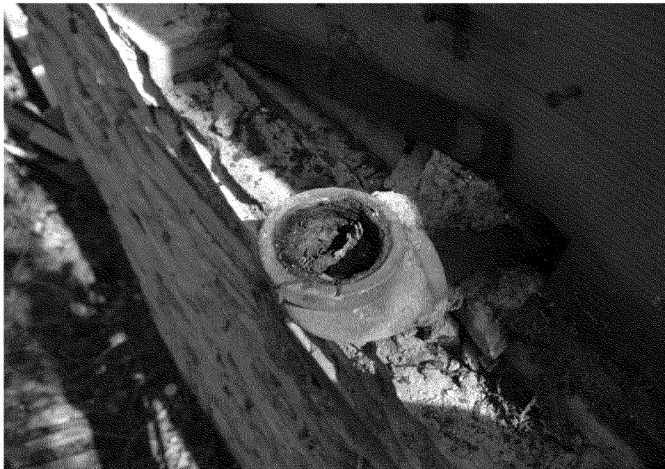
Figure 19. Vent pipe (broken off) in the bathroom. Photograph by Exponent on March 7, 2014.
