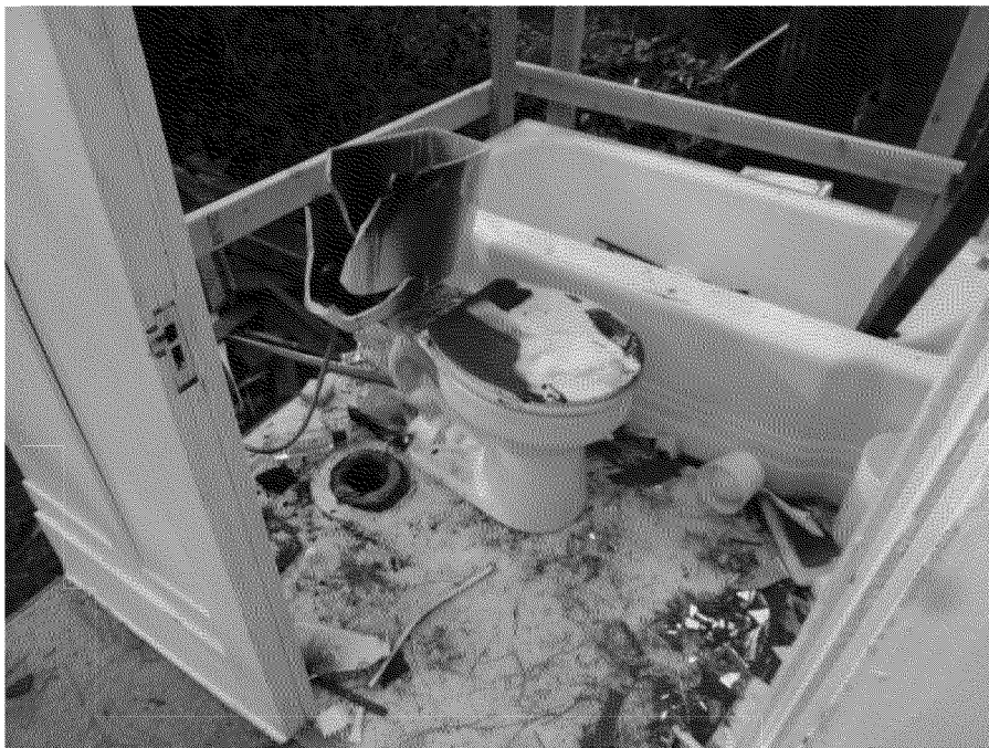
Figure 59. Monitoring point #15 after removal of the toilet. Photograph by Exponent on March 21, 2014.
