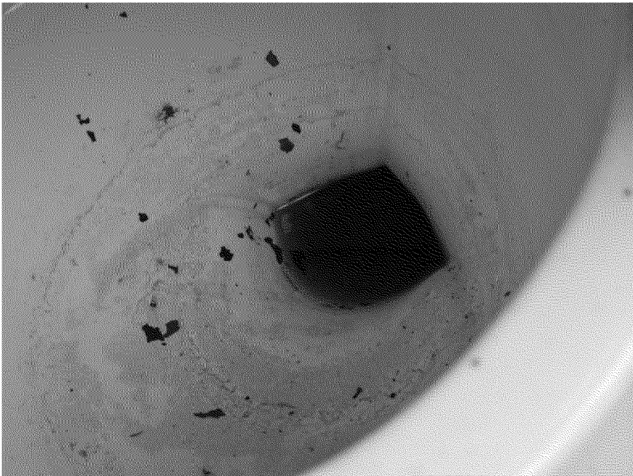
Figure 50. Low water level in the bathroom toilet bowl three days after explosion. Photograph by Exponent on March 6, 2014.
