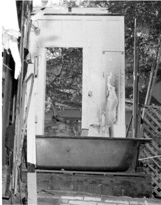
Figure 13. Fire pattern on bathroom wall, looking South from [Redacted] Photograph by Exponent on March 7, 2014.
