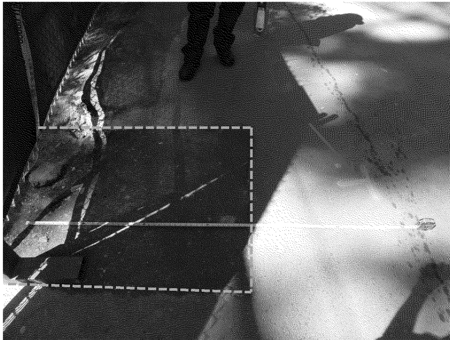
Figure 35. Relative location of cold asphalt patch for gas service tee (dashed yellow lines) and sewer lateral tap-in connection to sewer main (green arrow) for subject residence. Residence is to the left in photograph. Photograph by Exponent on March 11, 2014.
