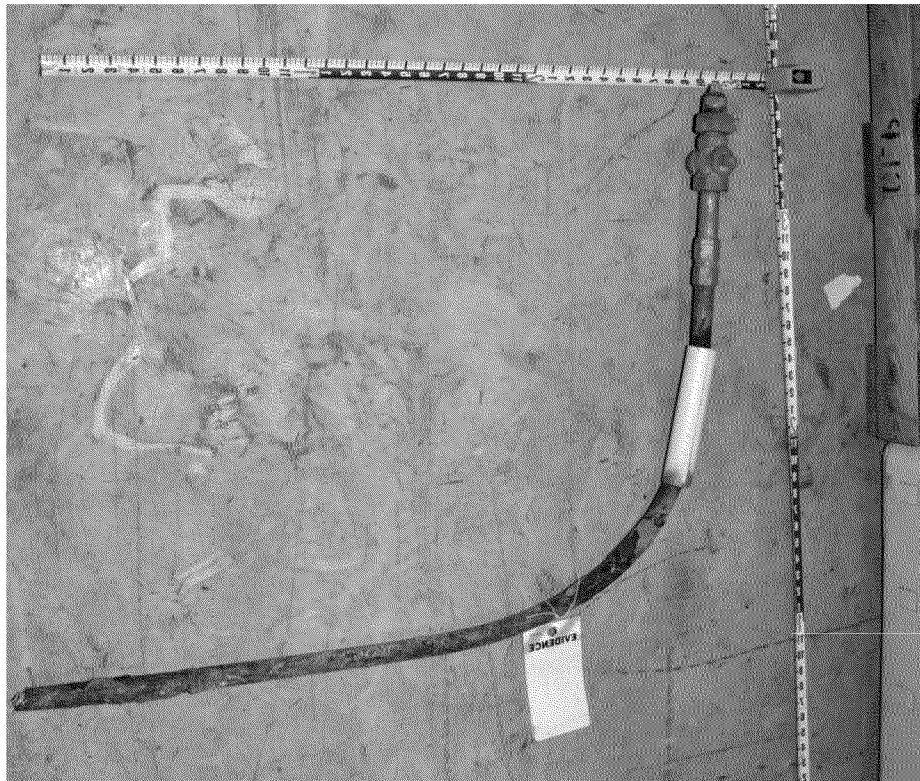
Figure 23. Portion of the gas service line to incident house. Photograph by Exponent on March 10, 2014.
