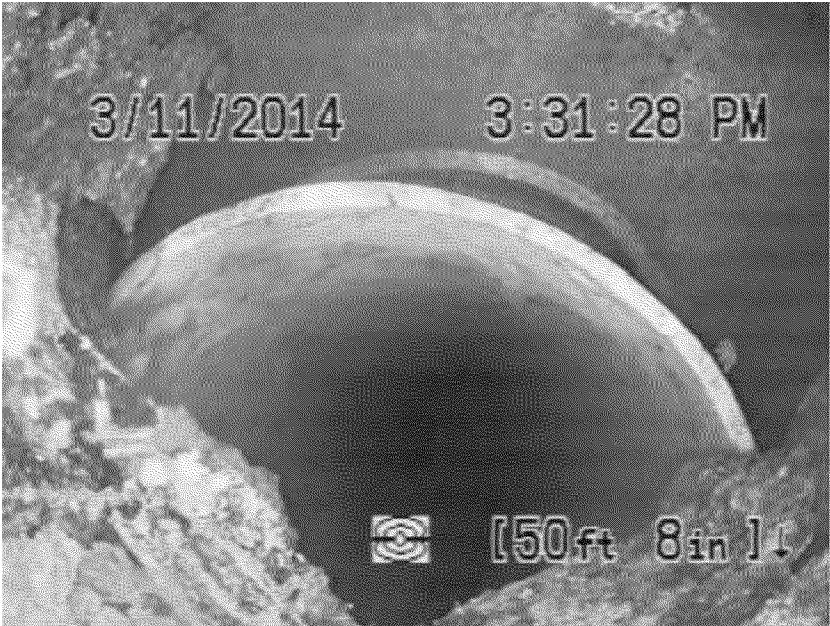
Figure 42. Dislocated joint between an apparently white plastic pipe and cast iron sewer lateral. Source: FES.
