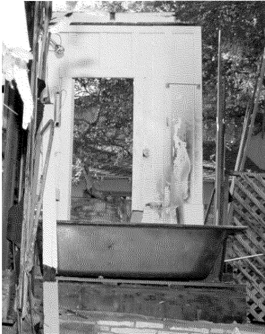
Figure 13. Fire pattern on bathroom wall, looking South from 3rd Avenue. Photograph by Exponent on March 7, 2014.
