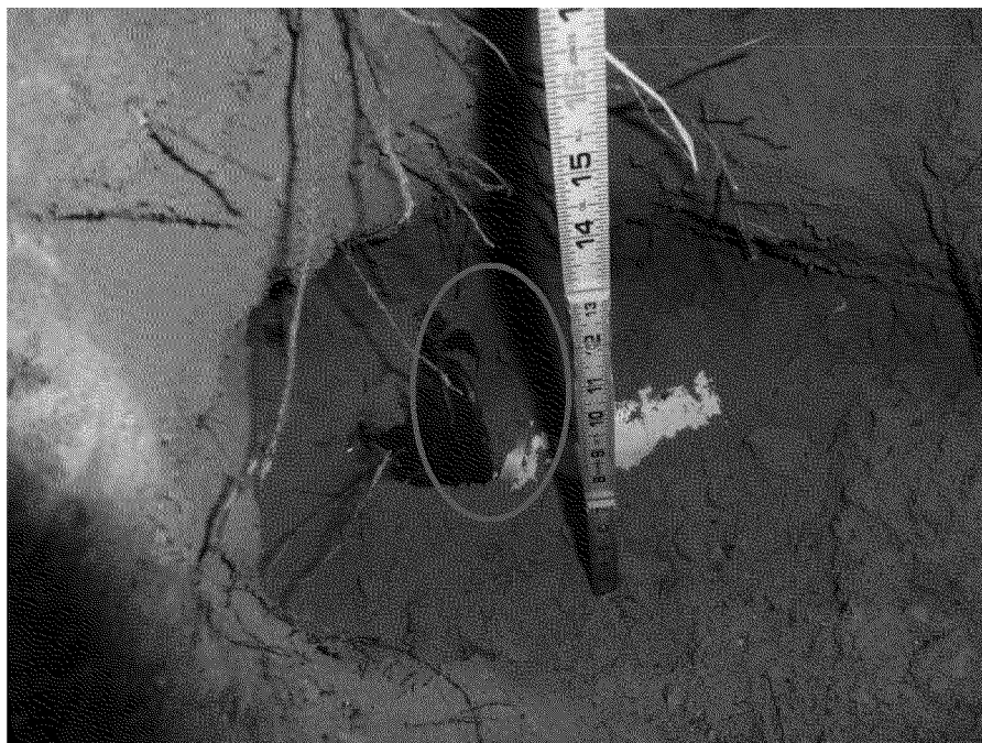
Figure 46. Sewer lateral offset joint (green oval), and white plastic segment of sewer lateral. Sand backfill surrounding sewer lateral. Photograph by Exponent on March 21, 2014.
