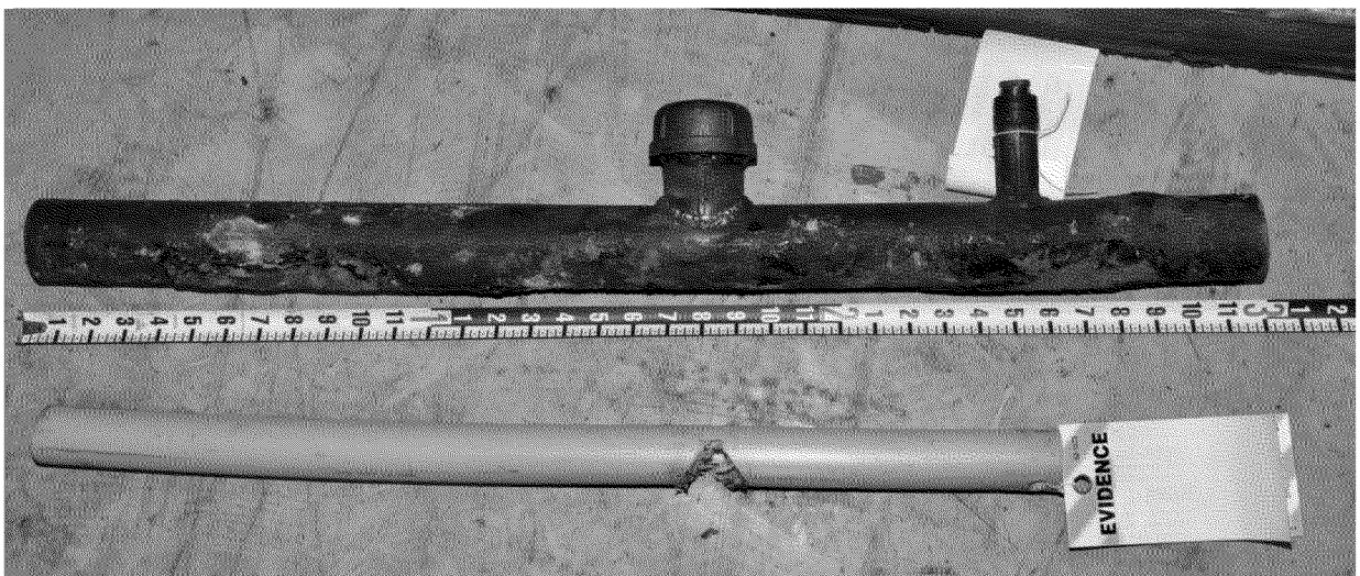
Figure 27. Portion of the gas main along 3 rd Avenue. Steel pipe (top) with welded fittings and plastic pipe insert. Photograph by Exponent on March 10, 2014.
