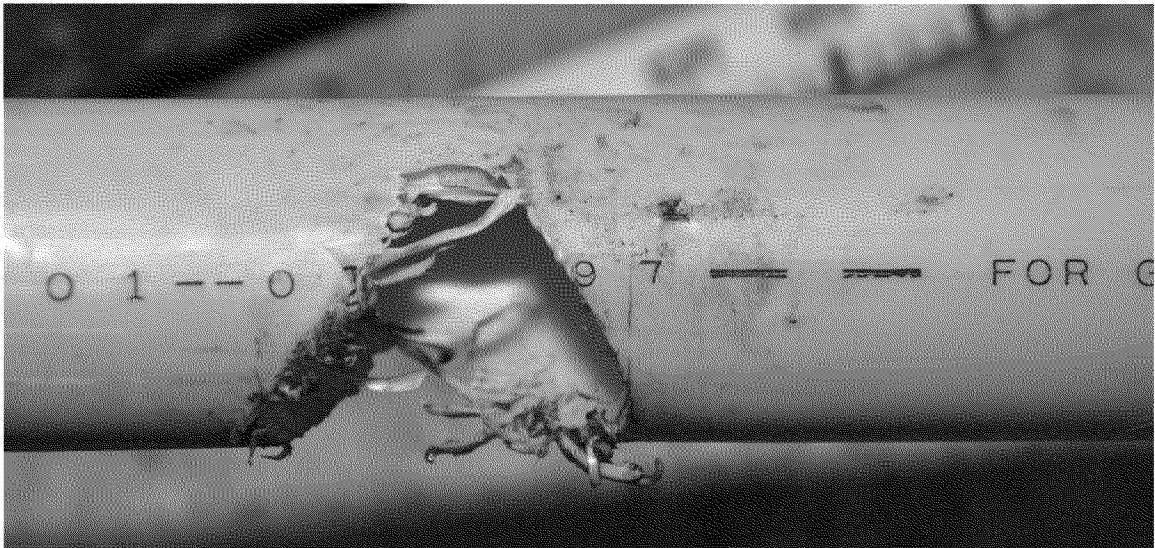
Figure 30. Close-up of the visible portion of the date code on the plastic pipe. Photograph by Exponent on March 10, 2014.
