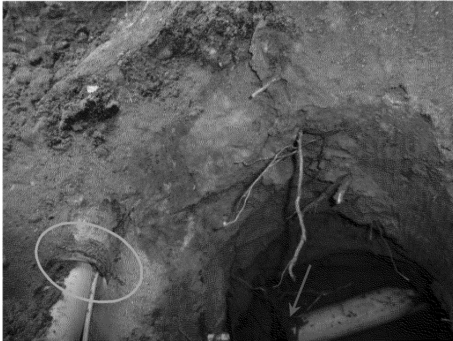
Figure 47. End of annular space in gas main along 3 rd Avenue (yellow oval) in vicinity of sewer lateral offset joint (green arrow). Photograph by Exponent on March 21, 2014.
