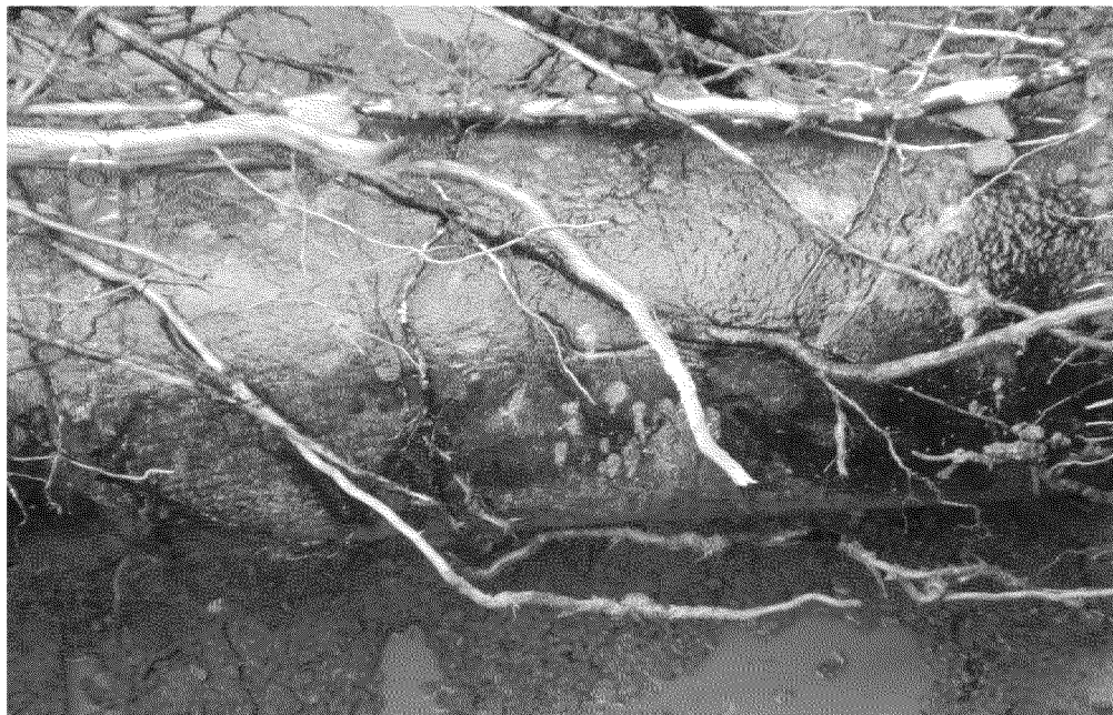
Figure 4. RWVIM-74-13 (Atascadero) (Tape coating damage)
