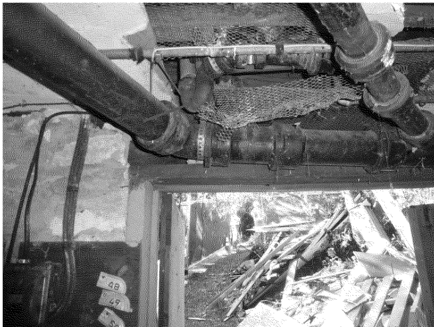
Figure 41. Multiple connections to building sewer system inside residence. Arrow indicates plumbing trap. Photograph from inside residence's basement. Photograph by Exponent on March 11, 2014.
