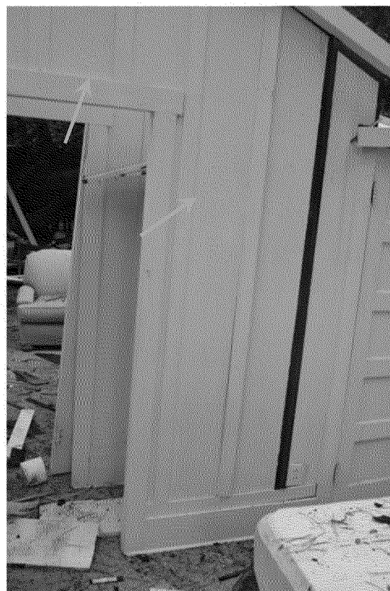
Figure 11. Interior walls and furniture. An unburned couch in the living room is visible in the background and the corner of an unburned mattress is visible in the foreground. Yellow arrows indicate some areas of wall blistering. Photograph by Exponent on March 6, 2014.
