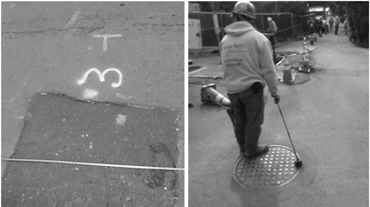
Figure 55. Example monitoring points outside of residence. Monitoring point #3 (left) near excavation performed by PG&E at gas service tee for residence. Monitoring point #19 (right) at sewer manhole near the intersection of Red Redacted Photographs by Exponent on March 21, 2014.
