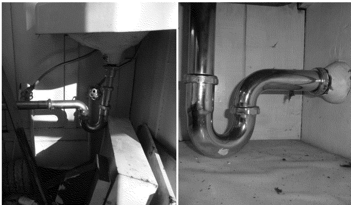
Figure 48. Plumbing traps at bathroom sink (left) and kitchen sink (right). Photographs by Exponent on March 11, 2014.
