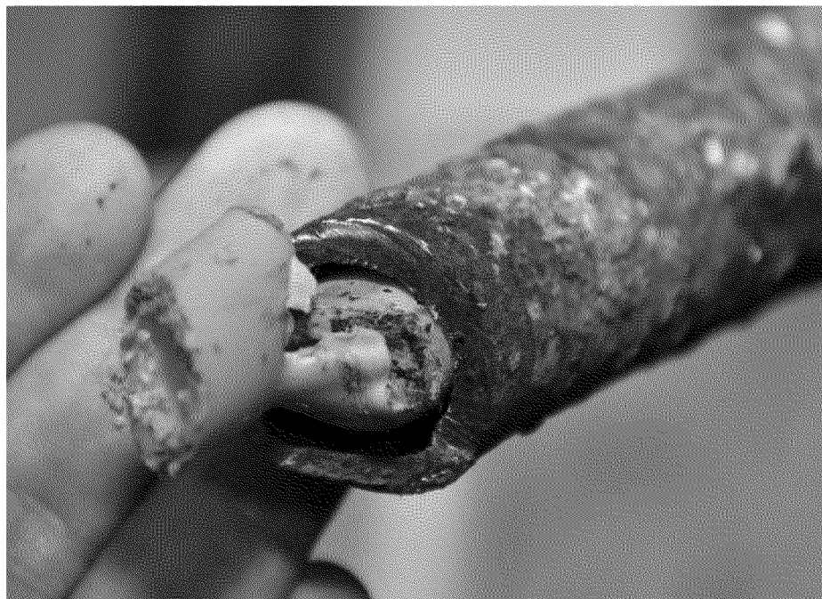
Figure 24. Close-up of the cut end of the gas service line. Photograph by Exponent on March 10, 2014.
