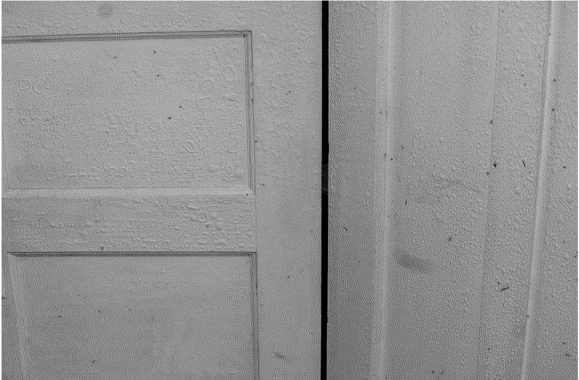
Figure 12. Close-up of the paint blistering on bedroom wall and door. Photograph by Exponent on March 7, 2014.
