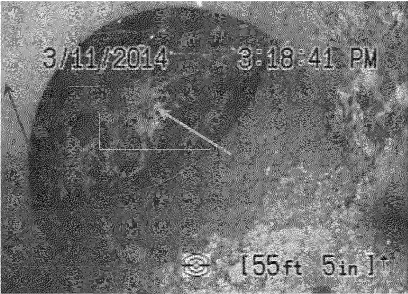
Figure 43. Sewer lateral joint offset at connection between white plastic pipe segment (green arrow) and apparent cast iron pipe (yellow arrow). Source: FES.
