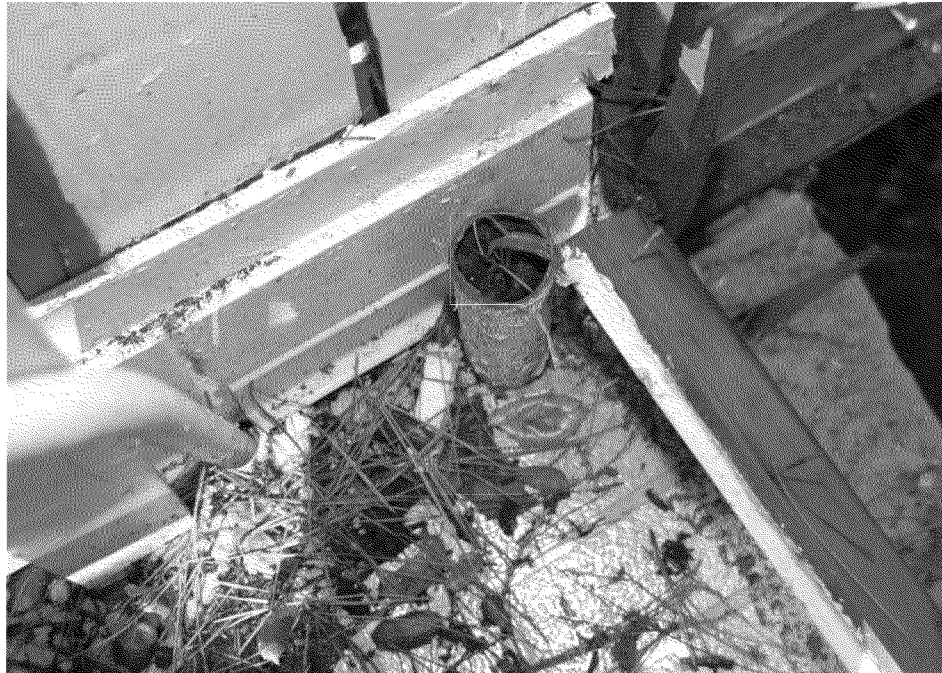
Figure 18. Sewer vent pipe (broken off) in the laundry room. Photograph by Exponent on March 7, 2014.
