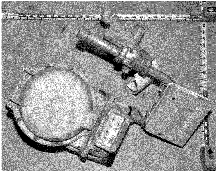
Figure 22. Regulator meter set removed from incident house. Photograph by Exponent on March 10, 2014.
