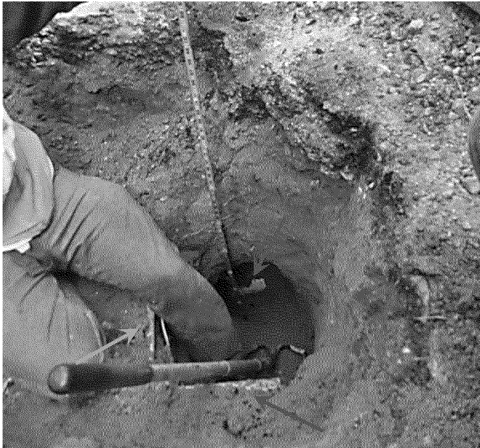
Figure 45. Excavation to expose sewer lateral at subject residence in the vicinity of gas service tee. Yellow arrow indicates gas main along [Redacted] Red arrow indicates gas service line. Green arrow indicates sewer lateral. Photograph by Exponent on March 21, 2014.
