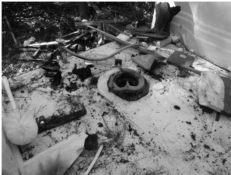
Figure 39. Toilet removed to allow for insertion of sewer push camera. Photograph by Exponent on March 11, 2014.
