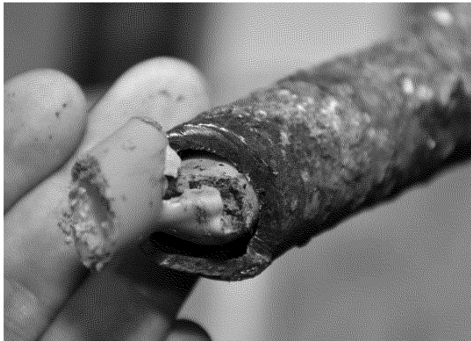
Figure 24. Close-up of the cut end of the gas service line. Photograph by Exponent on March 10, 2014.
