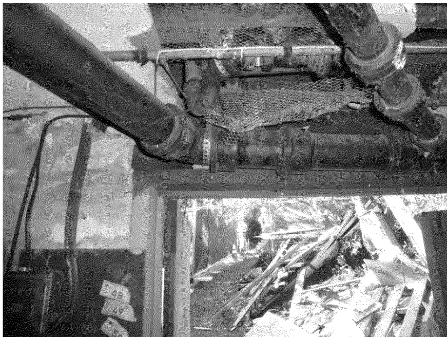
Figure 41. Multiple connections to building sewer system inside residence. Arrow indicates plumbing trap. Photograph from inside residence's basement. Photograph by Exponent on March 11, 2014.
