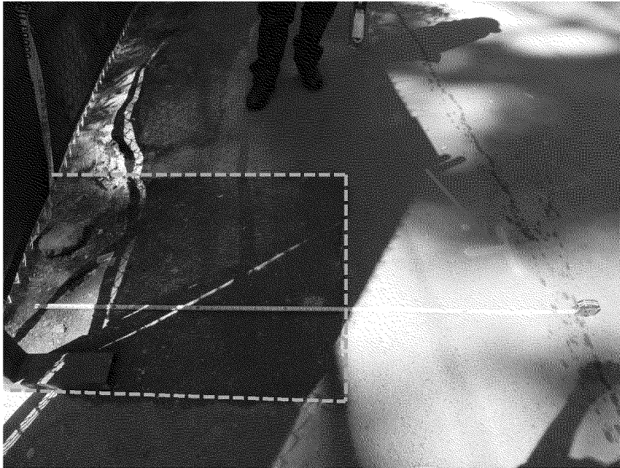
Figure 35. Relative location of cold asphalt patch for gas service tee (dashed yellow lines) and sewer lateral tap-in connection to sewer main (green arrow) for subject residence. Residence is to the left in photograph. Photograph by Exponent on March 11, 2014.
