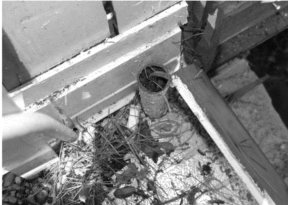
Figure 18. Sewer vent pipe (broken off) in the laundry room. Photograph by Exponent on March 7, 2014.
