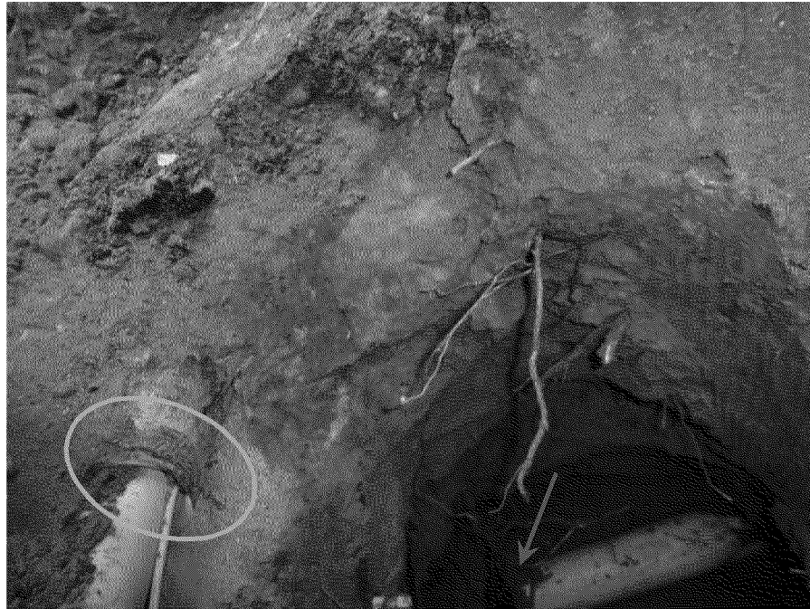
Figure 47. End of annular space in gas main along 3 rd Avenue (yellow oval) in vicinity of sewer lateral offset joint (green arrow). Photograph by Exponent on March 21, 2014.
