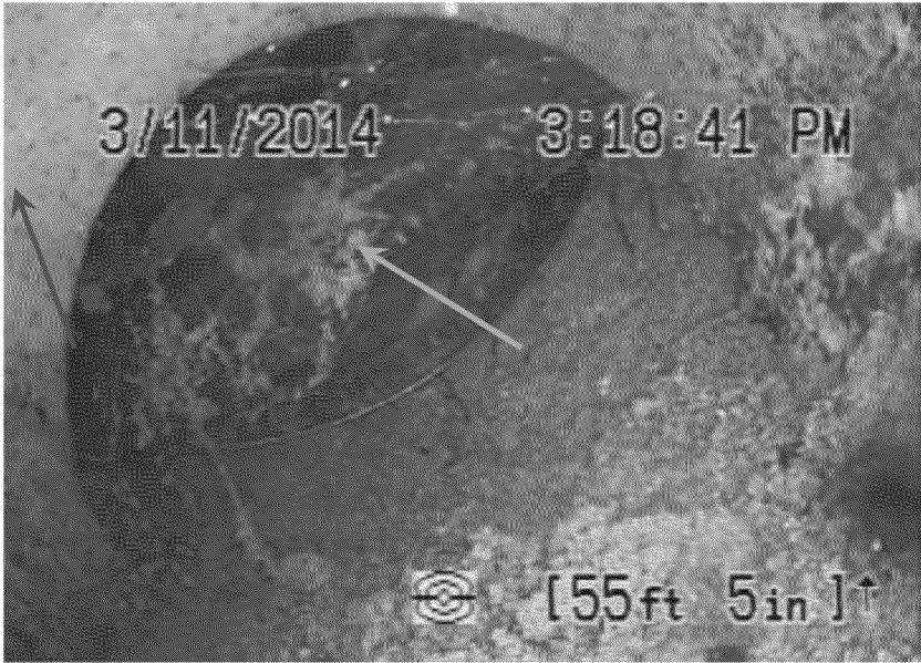
Figure 43. Sewer lateral joint offset at connection between white plastic pipe segment (green arrow) and apparent cast iron pipe (yellow arrow). Source: FES.
