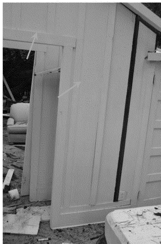
Figure 11. Interior walls and furniture. An unburned couch in the living room is visible in the background and the corner of an unburned mattress is visible in the foreground. Yellow arrows indicate some areas of wall blistering. Photograph by Exponent on March 6, 2014.
