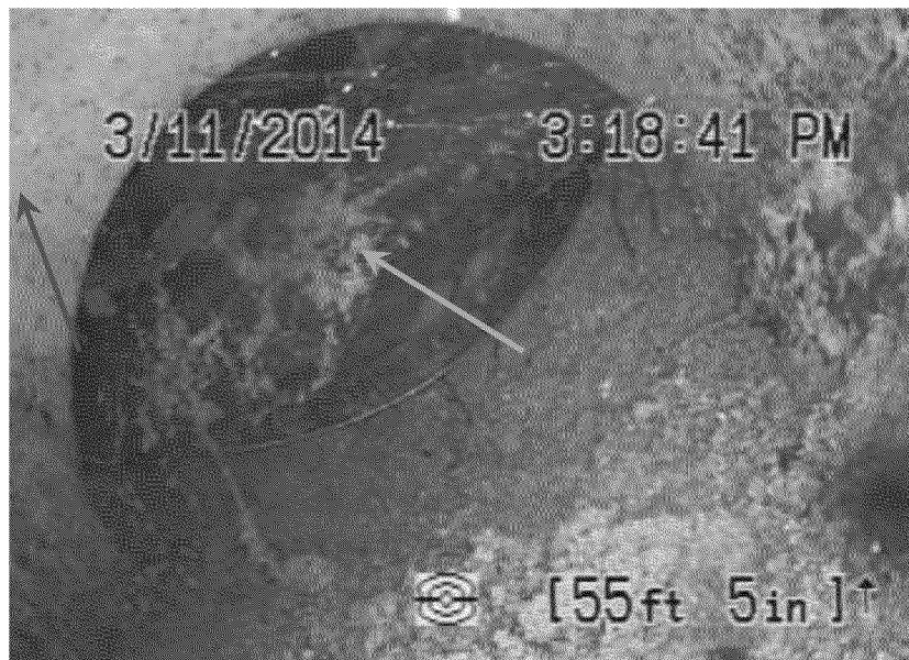
Figure 43. Sewer lateral joint offset at connection between white plastic pipe segment (green arrow) and apparent cast iron pipe (yellow arrow). Source: FES.
