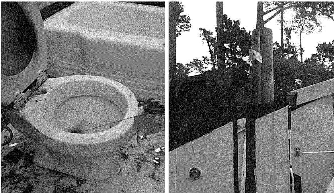
Figure 57. Example monitoring points at the residence's first floor. Monitoring point #15 (left) at the toilet. Monitoring point #18 (right) at bathroom vents. Photographs by Exponent on March 21, 2014.
