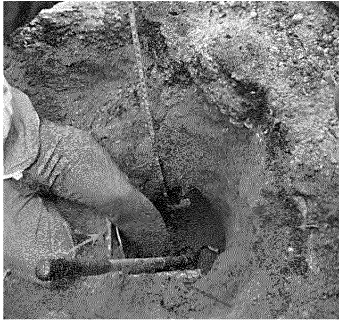
Figure 45. Excavation to expose sewer lateral at subject residence in the vicinity of gas service tee. Yellow arrow indicates gas main along Re Redacted Red arrow indicates gas service line. Green arrow indicates sewer lateral. Photograph by Exponent on March 21, 2014.
