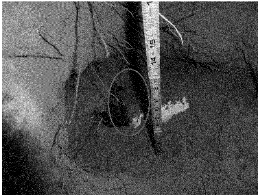
Figure 46. Sewer lateral offset joint (green oval), and white plastic segment of sewer lateral. Sand backfill surrounding sewer lateral. Photograph by Exponent on March 21, 2014.
