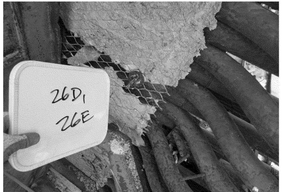
Sample 26D & 26E Refractory - Boiler 1
