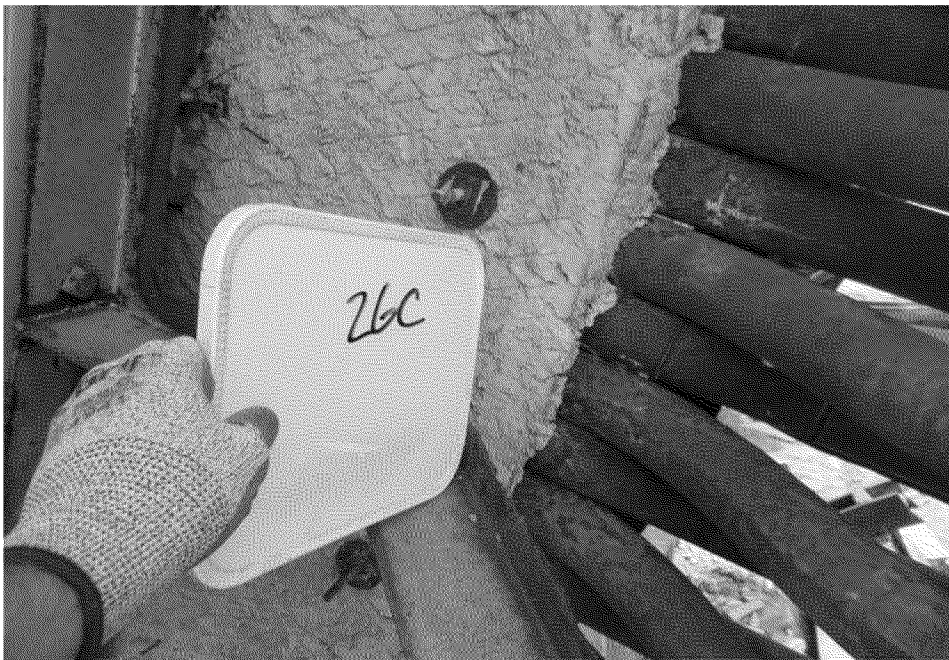
Sample 26C Refractory - Boiler 1
