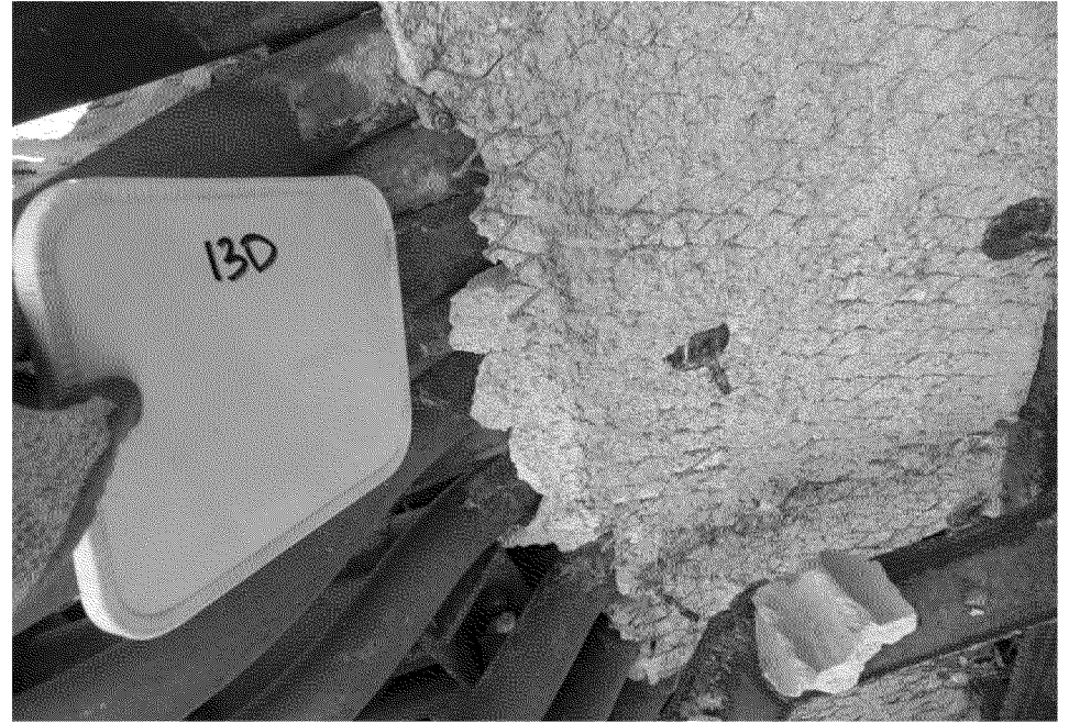
Sample 13D Refractory - Boiler 2
