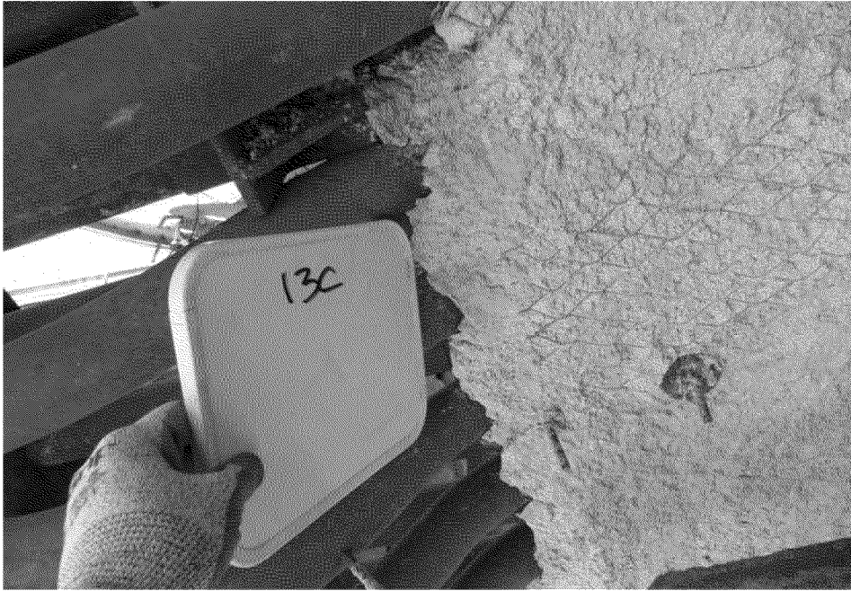
Sample 13C Refractory - Boiler 2
