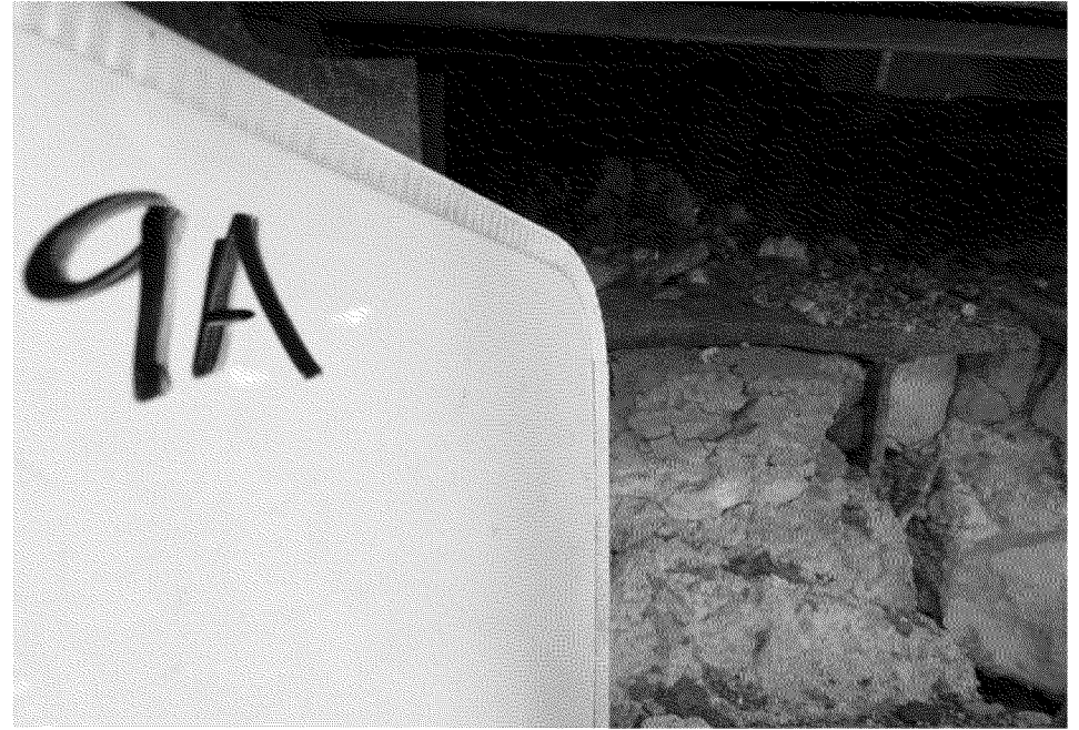
Sample 9A Misc. Tile - Boiler 2
