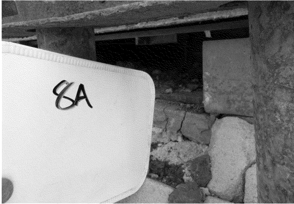
Sample 8A Boiler Mortar - Boiler 2
