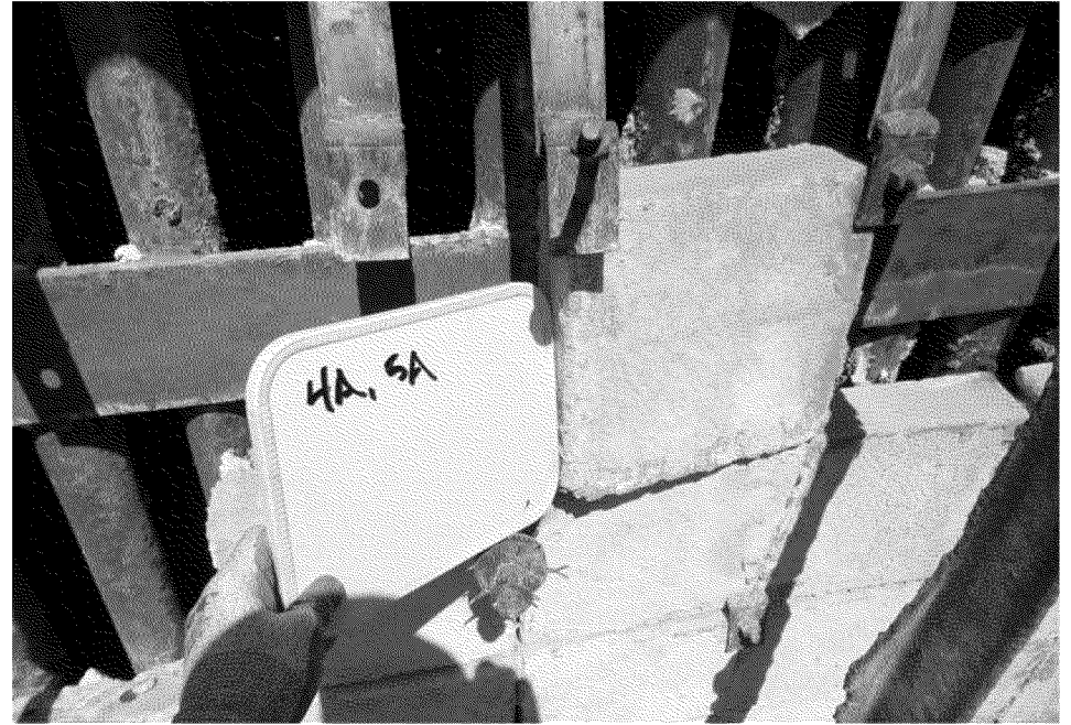
Sample 5A 12 Inch Tile Grout - Boiler 4
