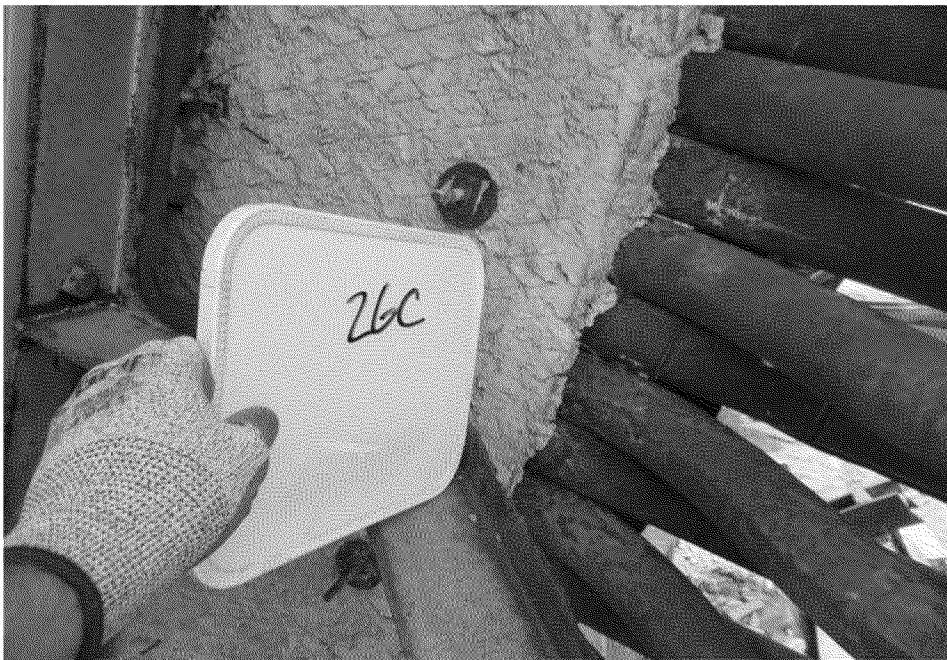
Sample 26C Refractory - Boiler 1
