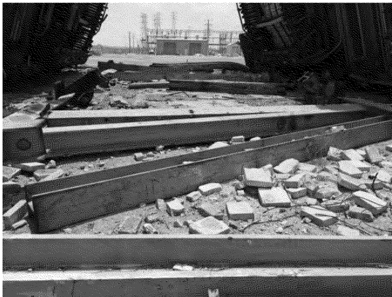
Debris Between Boiler Structures (View Looking South)
