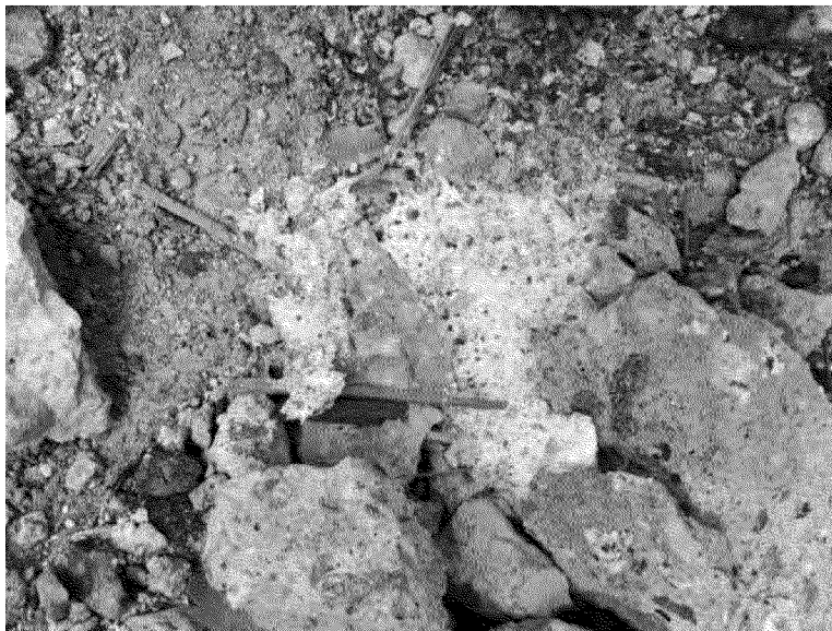
TSI Debris Between Boiler Structures (Closeup View)
