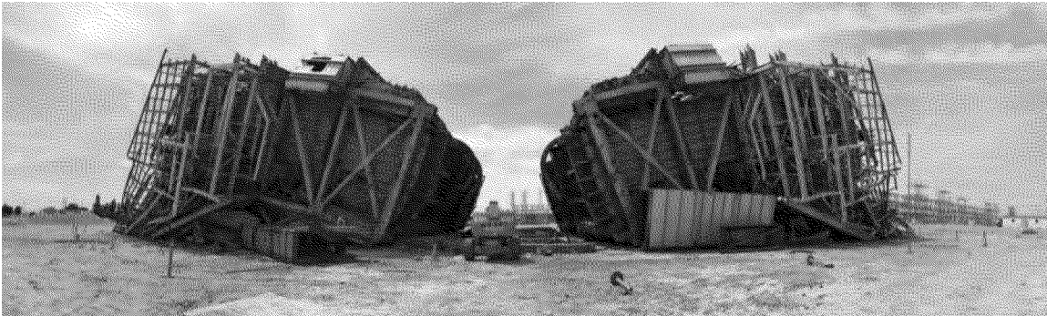
Felled Boiler Structures (View Looking South)
