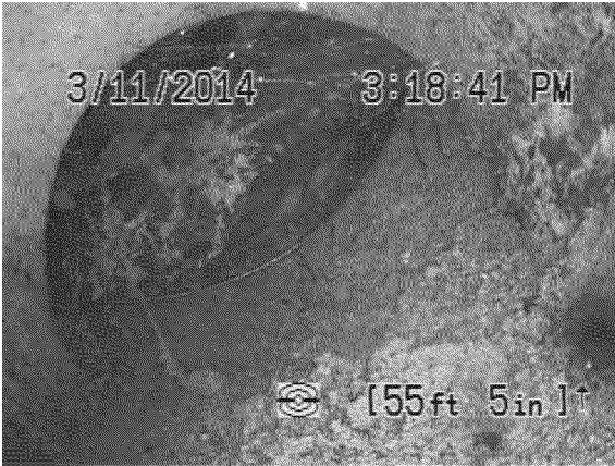
Figure 7. Lateral bend 55 ft. from entry
