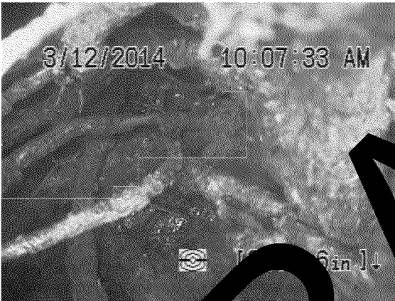
Figure 9. Lateral blocked by roots
