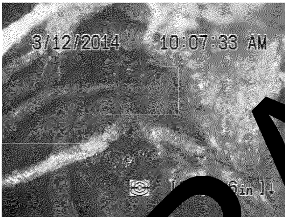
Figure 9. Lateral blocked by roots
