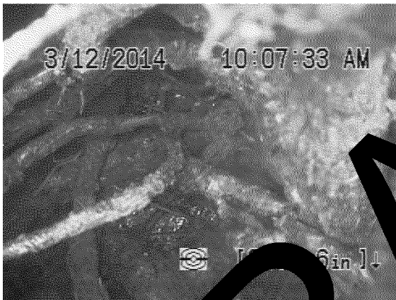
Figure 9. Lateral blocked by roots
