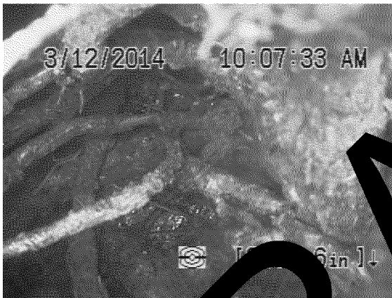
Figure 9. Lateral blocked by roots
