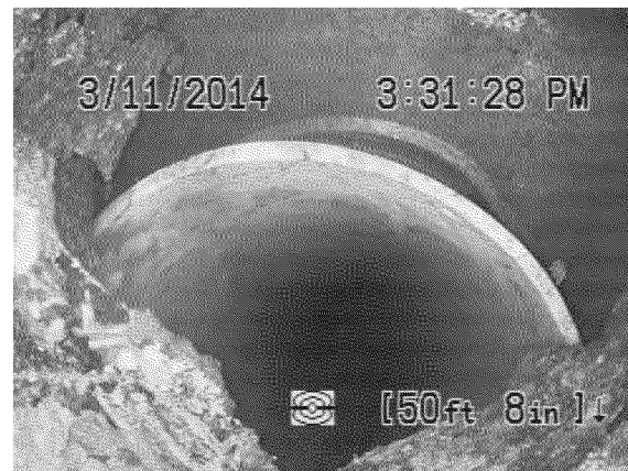
Figure 6. Offset joint 50 ft. from entry on property
