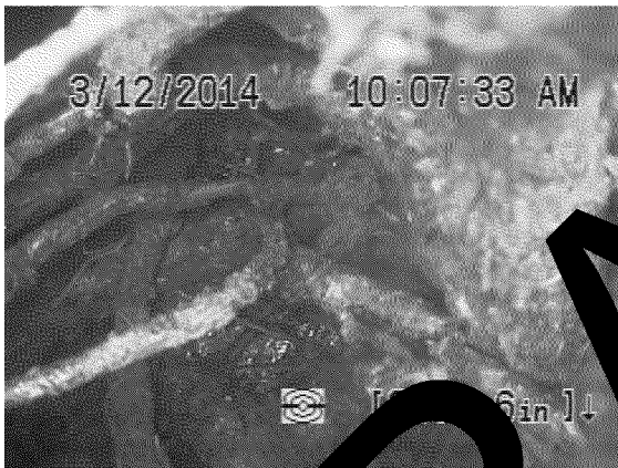
Figure 9. Lateral blocked by roots
