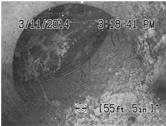
Figure 7. Lateral bend 55 ft. from entry
