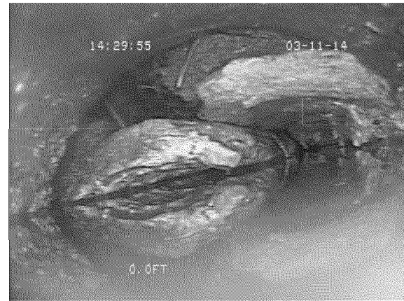
Figure 8. Collapsed main and water in sag
