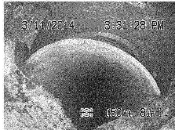
Figure 6. Offset joint 50 ft. from entry on property
