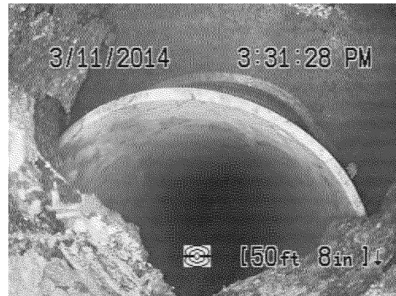
Figure 6. Offset joint 50 ft. from entry on property
