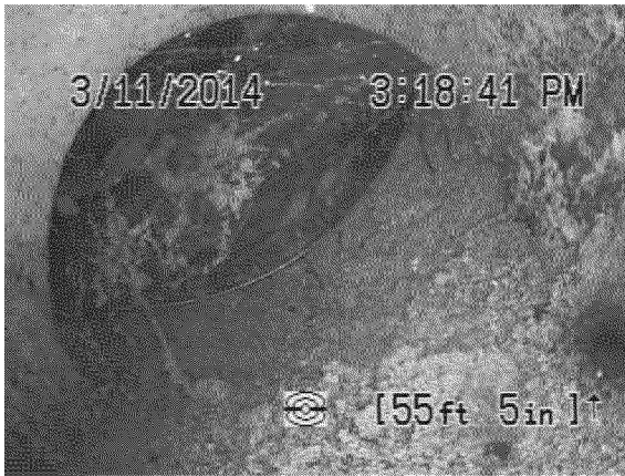
Figure 7. Lateral bend 55 ft. from entry
