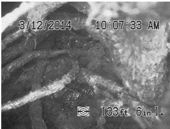
Figure 9. Lateral blocked by roots
