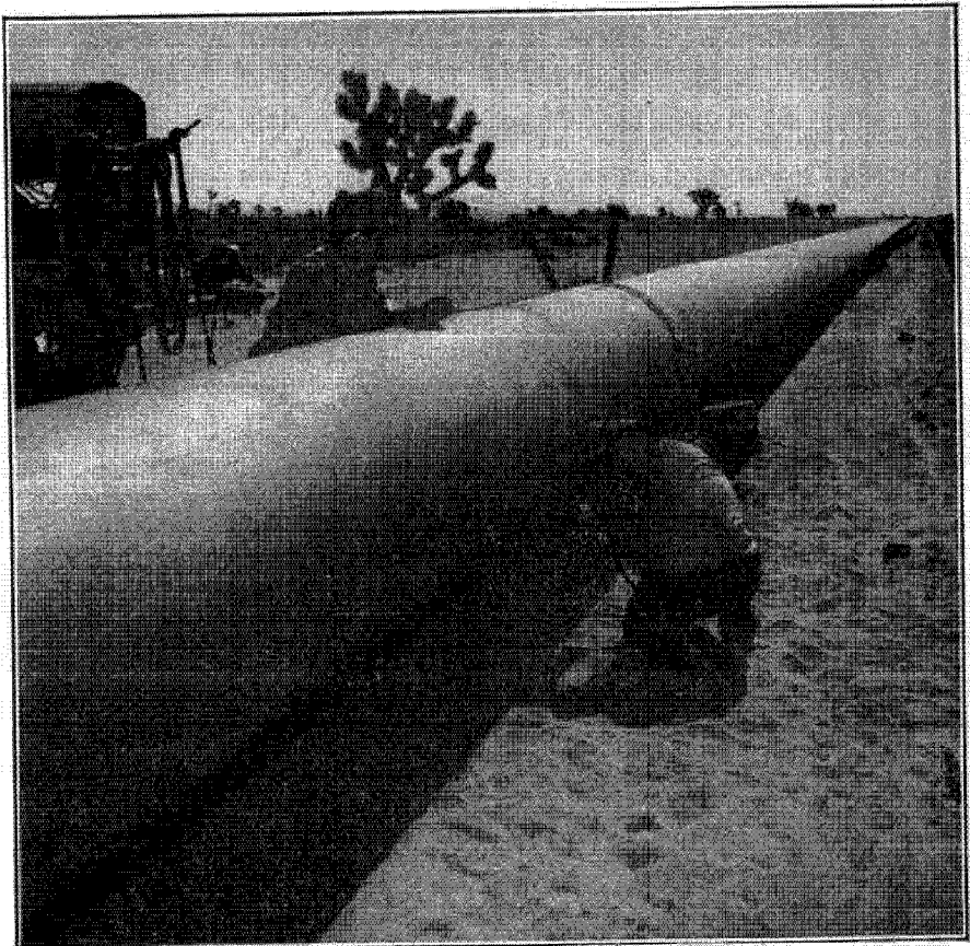
This picture of the P. G. and E.'s pipeline was taken on the Mojave Desert. The size of the main can be gauged by comparison with the workmen.
