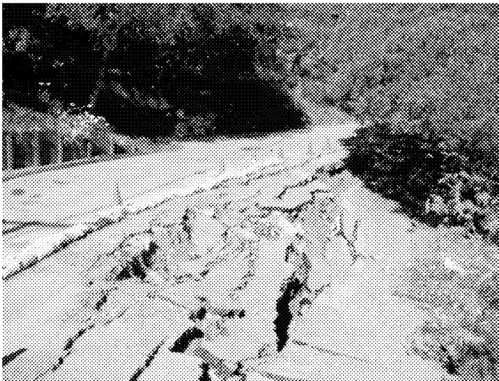
Figure 4. Lateral spreading caused by landsliding.
