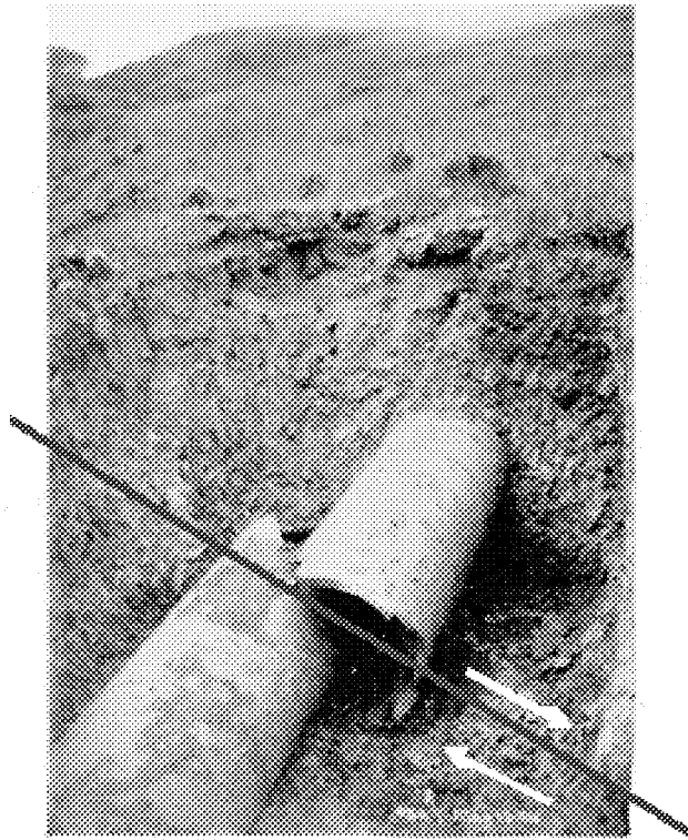
Fig. 1. 30" Pit Pipe. Detail of north end of break on view N2. E. on Map 13.
