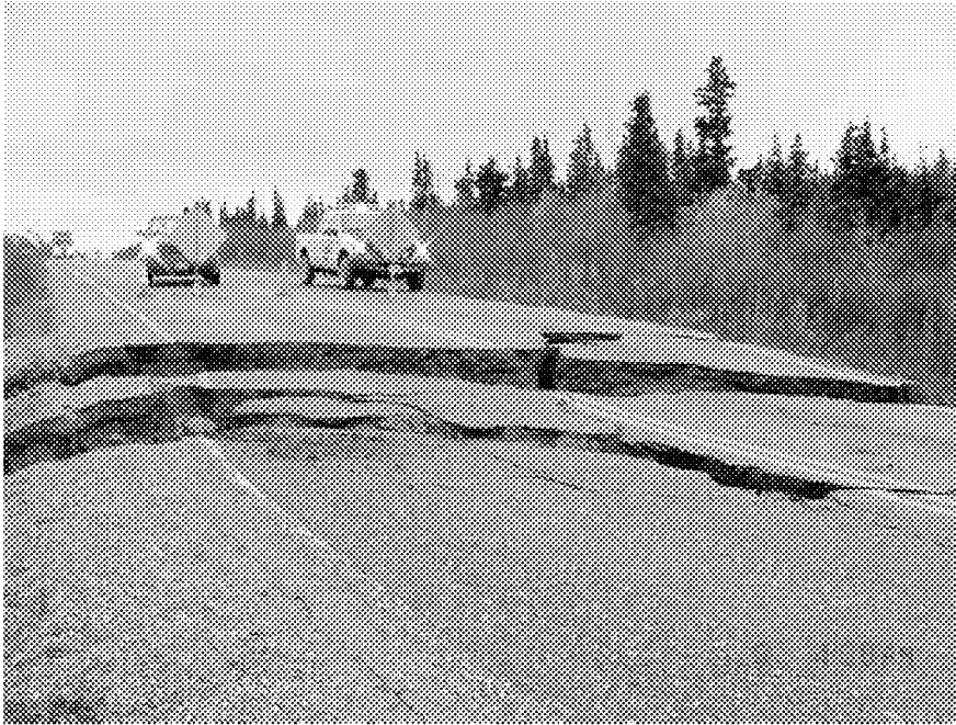
Figure 3. Lateral spreading caused by ground shaking.
