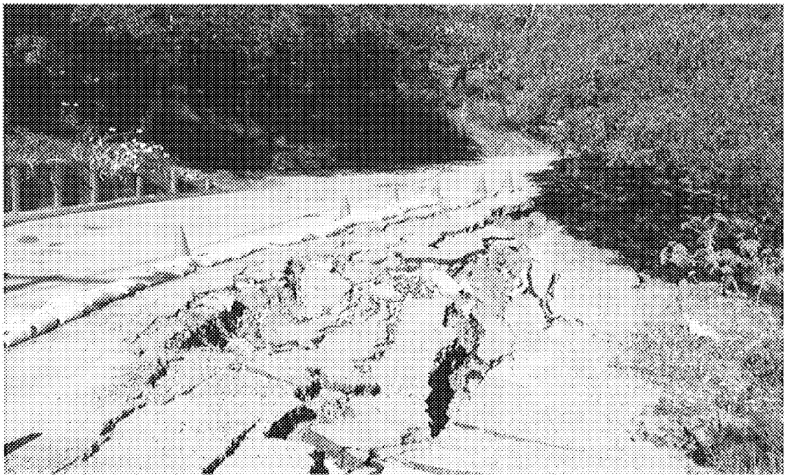
Figure 1 Lateral spreading Caused by Landslide
