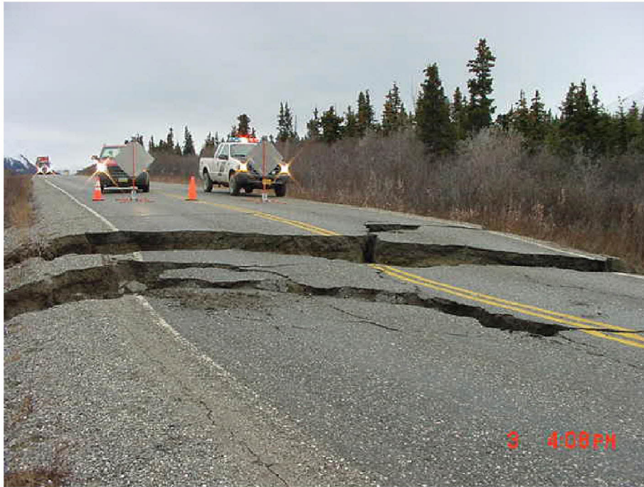
Figure 3. Lateral spreading caused by ground shaking.
