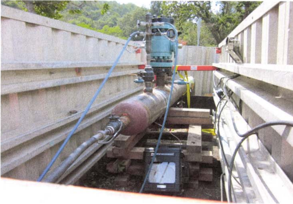
Test 022A-12 test 3 test head at Loc. A with test hoses attached
