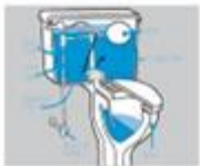
Water in the overflow pipe could also be caused by a pinhole in the float or a worn washer on the inlet line.
