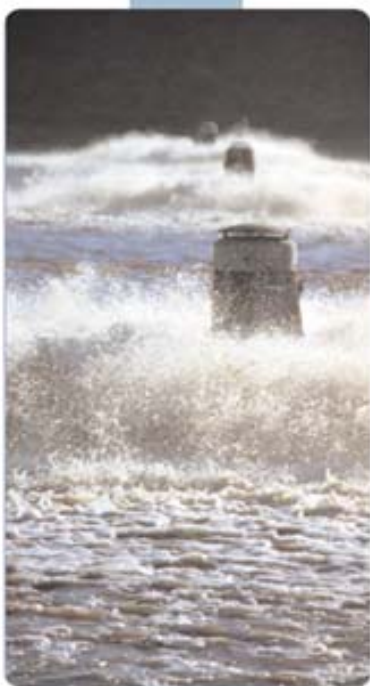
Aeration pond at the City of Riverbank wastewater facility. The Central Valley city, population 16,000, will save a projected $20,000 annually in energy costs through process improvements fully funded by the California Process Optimization Program.
