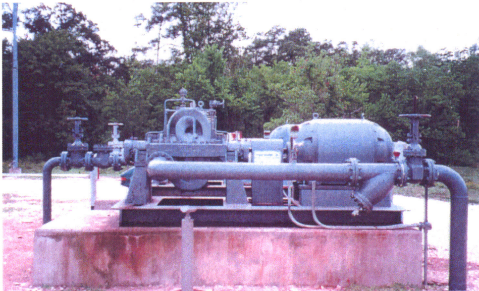
PHOTO 8: Water Injection Pump
