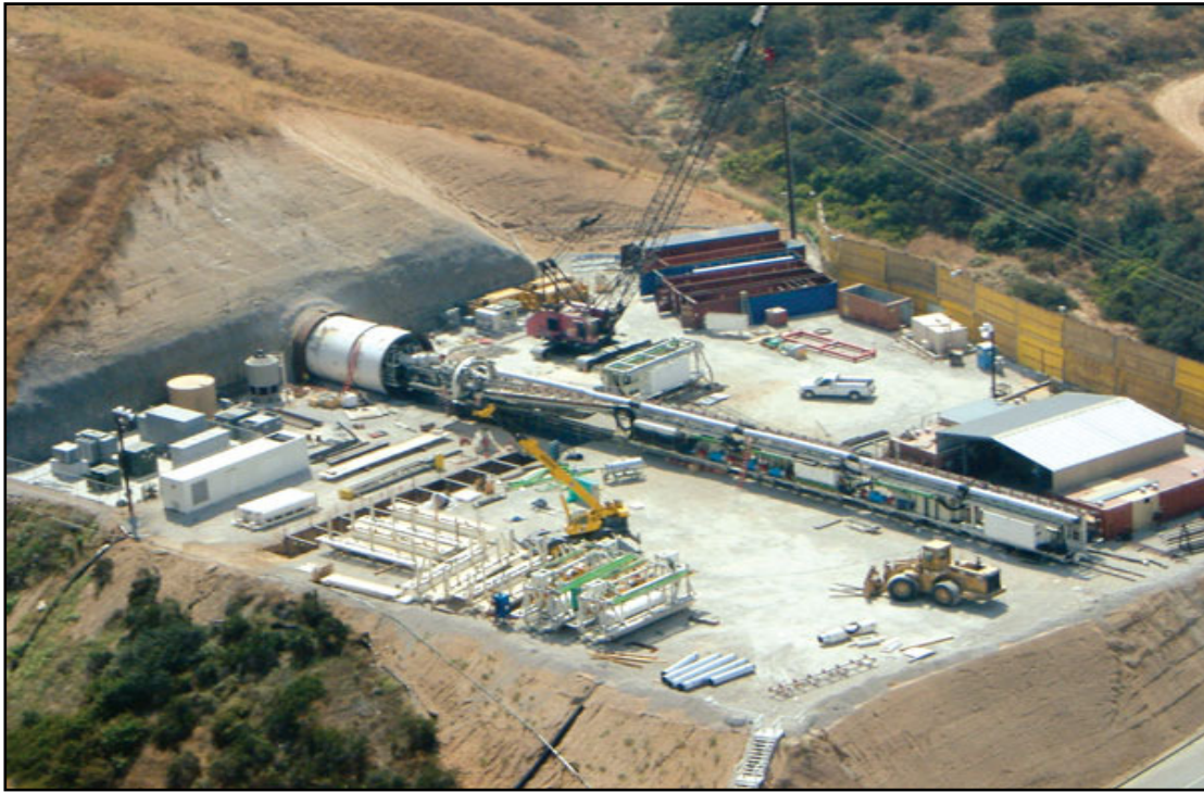
Photo 1: Assembly of the tunnel boring machine at the Strawberry Creek Portal. Source: Neufeld, 2007
