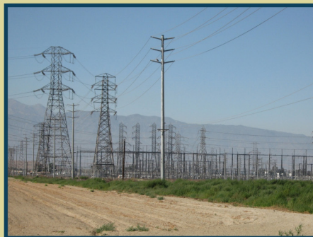
Mira Loma Substation
