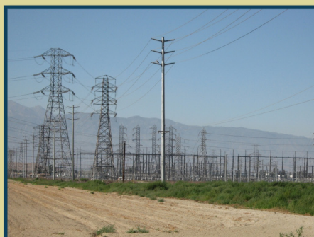
Mira Loma Substation
