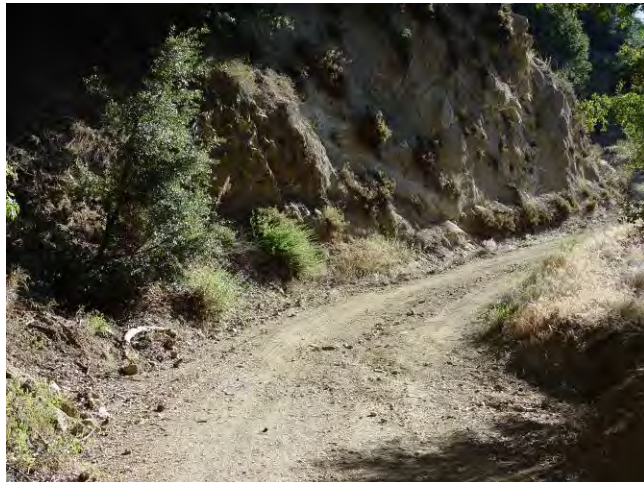
Steep road cut on the upslope. Non-native grasses can be seen along the right side of the road.
