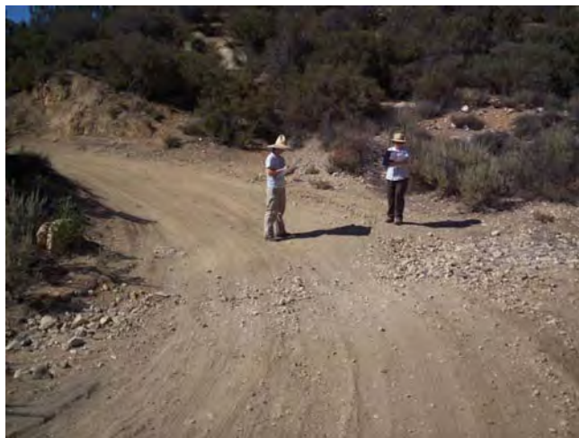
View along Lynx Gulch Road (4N18.2). Note well defined water channel across the road.
