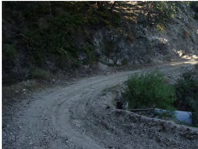
Road is narrow around curve and has steep cut into the upslope.
