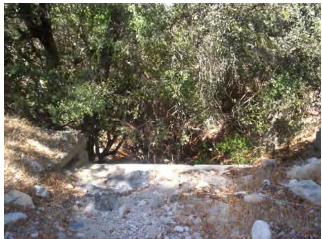
View towards downstream portion of tributary drainage. Note concrete spillway at center of photo.
