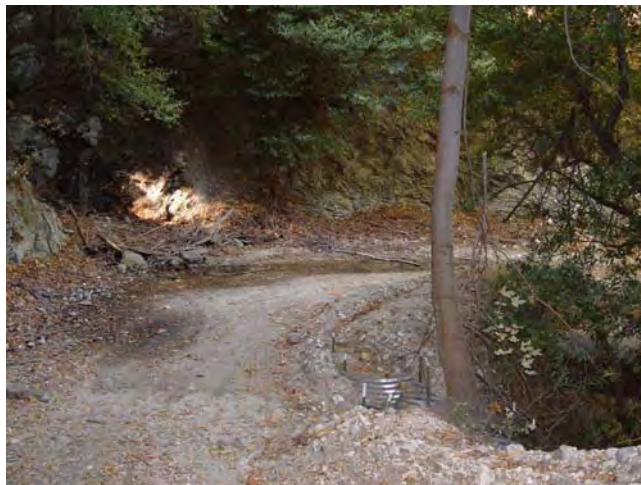
View along Shortcut Edison Road (2N23). Note seep at road edge in background.
