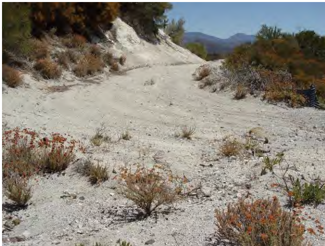
Note open exposed areas of sand and bedrock.
