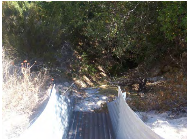
View down drainage. Note McCarthy drain in foreground and dense riparian vegetation in drainage.
