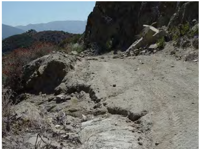
Note scour line and ruts from flow events.
