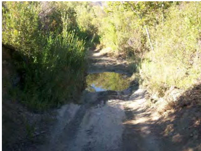
View along Lynx Gulch Road (4N18.2). Note ponded water in roadway.
