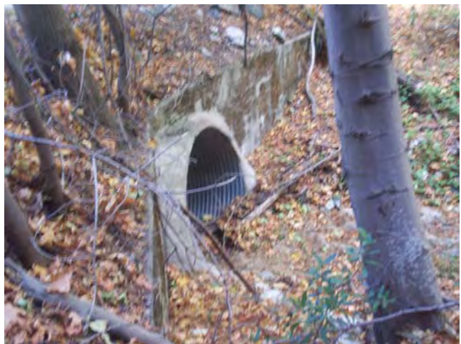
View of CMP located along downstream reach of tributary drainage as it bisects the road.
