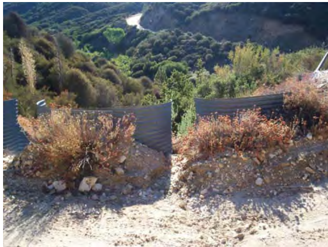
View down drainage. Note McCarthy drain and steep drop off.
