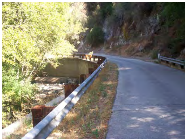
View along 2N25.1 across concrete bank wall with several CMPs underneath road. West Fork San Gabriel River visible just below bank wall.
