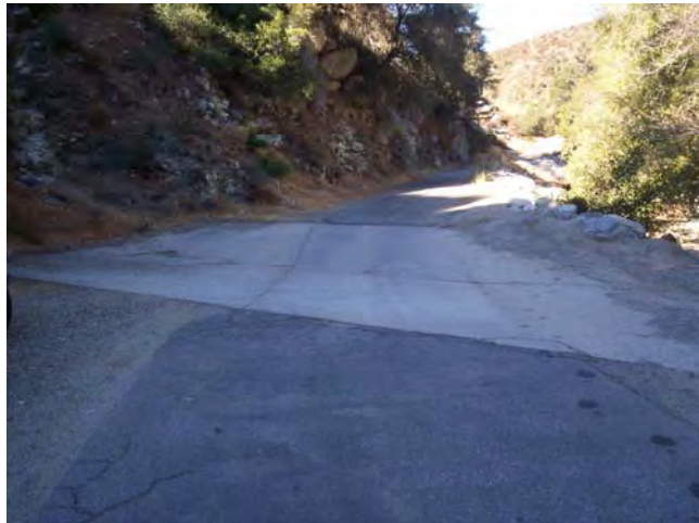
View along 2N25.1 across paved Arizona crossing. West Fork San Gabriel River occurs just along left side of photo.
