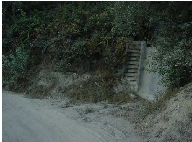
Note concrete barrier across drainage and dense riparian vegetation.
