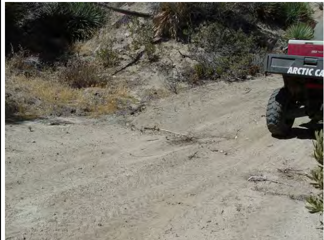
Faint scour line of drainage crossing road.
