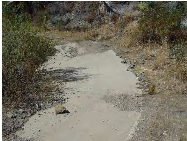
Decomposing asphalt with chamise chaparral encroaching.
