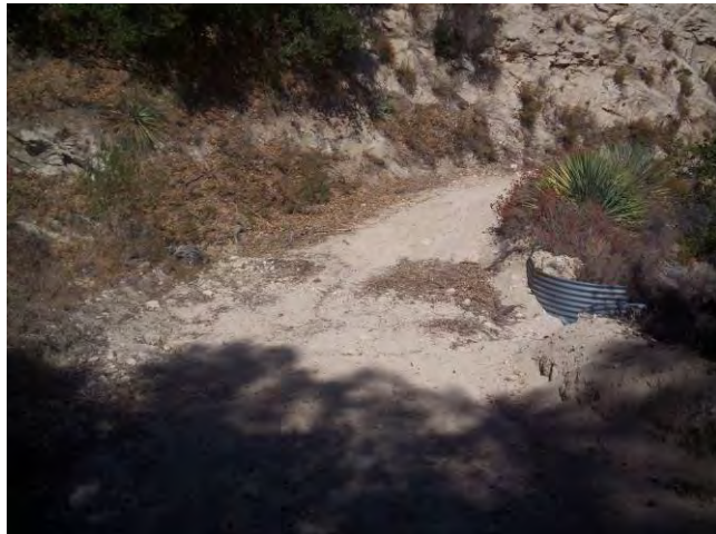
View along Edison/Fall Creek Road (3N27). Note scour line and McCarthy drain.
