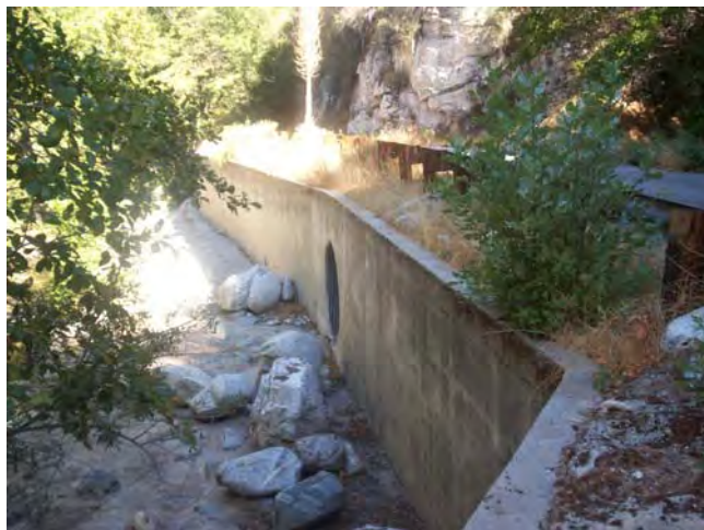
View of concrete bank wall with large CMP. This photo was taken at the eastern end of the crossing at this location. The concrete bank wall extends further west for approximately 100 feet and several more CMPs are present. The southern bank of the West Fork San Gabriel River is visible just below the concrete bank wall.
