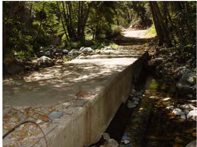
Note exposed rebar and deteriorated concrete at crossing. Note presence of perennial water.
