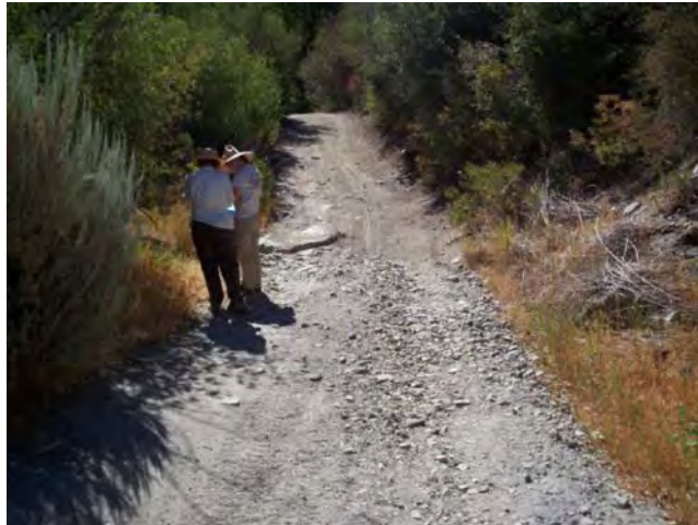
View along Monte Cristo Creek Road (3N23). Note debris on right side of road.
