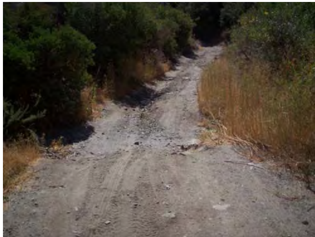
View along Monte Cristo Creek Road (3N23). Depression and rills in roadway indicate water flows in road during precipitation events.
