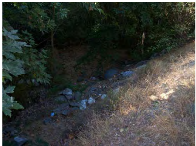
View along upstream portion of the tributary drainage at this location. This drainage parallels the road for approximately 100 feet before flowing through CMP located underneath road crossing.
