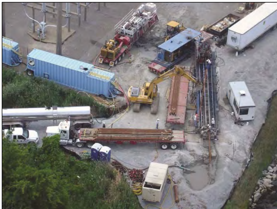
Figure A.1-8: Equipment Setup for a major HDD installation crossing a river (Source: Power Delivery Consultants, 2012)
