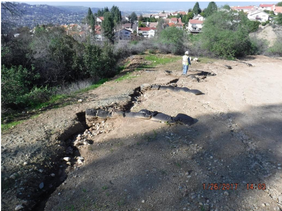
Figure 8: Erosion of access road at Tower 49-T2, Segment 8 Overhead. Photo courtesy of SCE.
