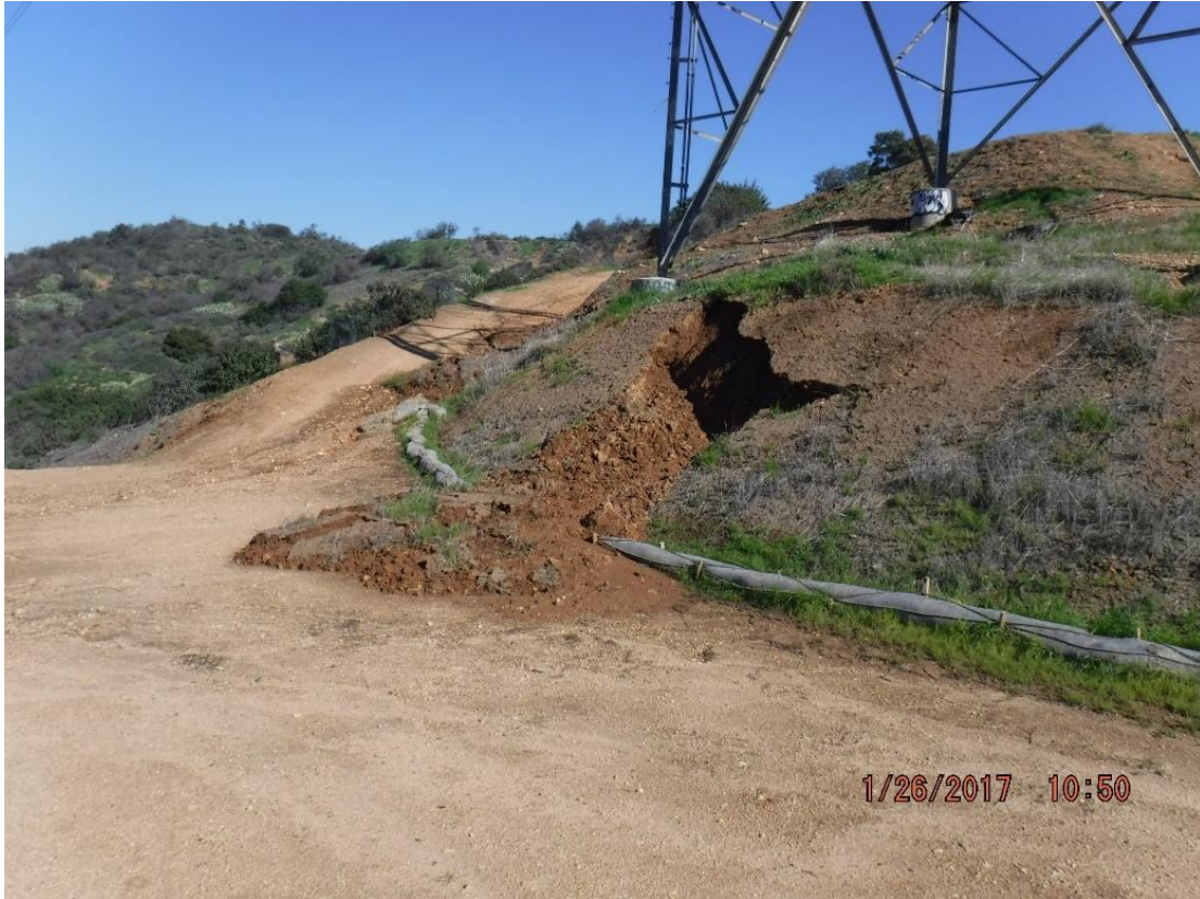
Figure 7: Erosion at Tower 45-T5, Segment 8 Overhead. Photo courtesy of SCE.
