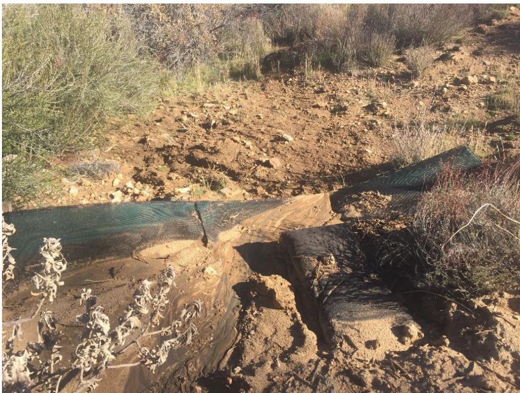
Figure 4: Off-site sedimentation and BMP failure observed at Tower 16, Segment 11.
