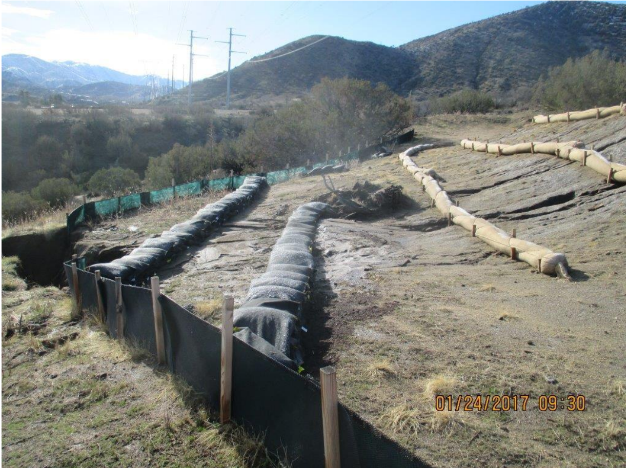
Figure 5: Rilling, gully, and sediment buildup at Tower 6 before maintenance, Segment 6. Photo courtesy of SCE.
